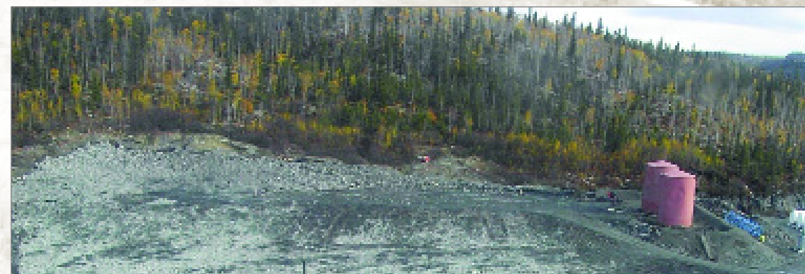
Larger boulders were used as final cover in the Tank Farm Area.
