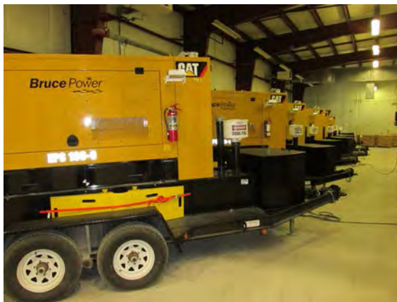
NPP emergency mitigating equipment includes portable emergency power generators.
