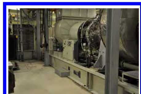
Emergency power generators are available to provide electrical power in the event the NPP becomes disconnected from the grid.
