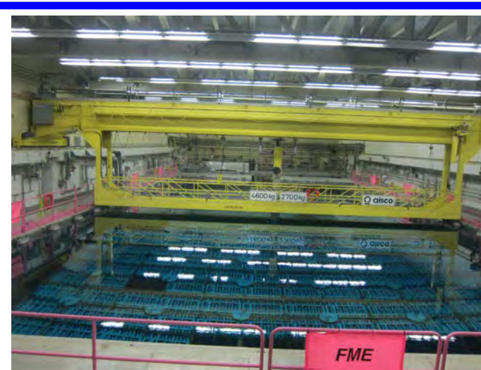
Irradiated fuel bays are designed to cool used fuel. After 6 to 10 years in wet storage, the nuclear fuel can be safely transferred to dry storage in concrete canisters.
