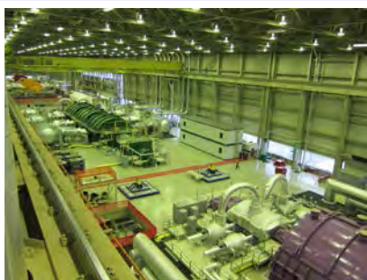
Turbine hall, located on the non-nuclear side of the Darlington NPP.
