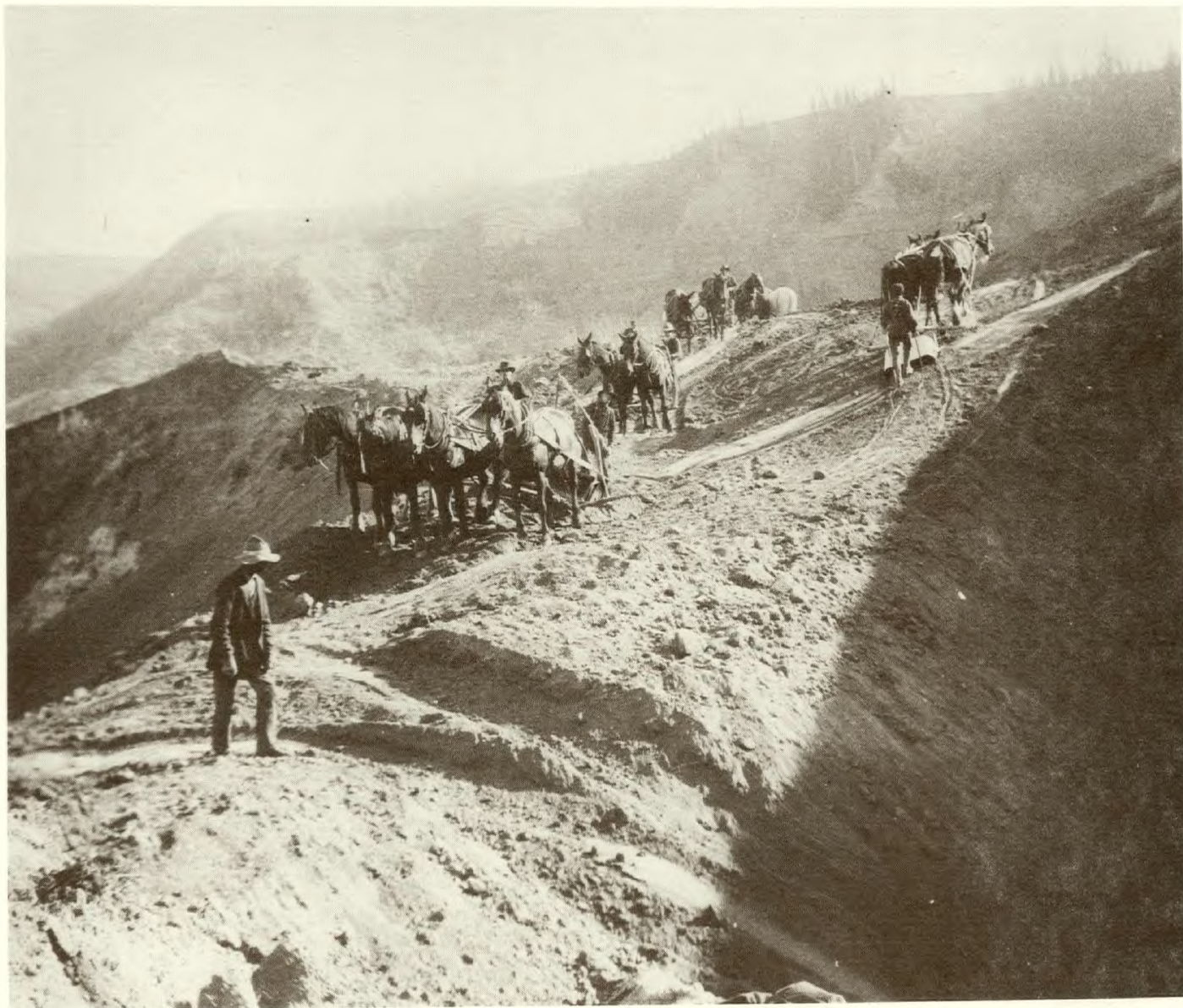
121. Railway grading, Alberta. According to the Canadian Annual Review for 1907, 5,800 miles of railroad were under contract between the Great Lakes and the Rocky Mountains. Included were 1,500 miles of the Canadian Northern, 1,400 miles of the Canadian Pacific, 1,000 miles of the Great Northern and 1,900 miles of the Grand Trunk Pacific. By September 1907, approximately 3,000 miles were actually under construction.
