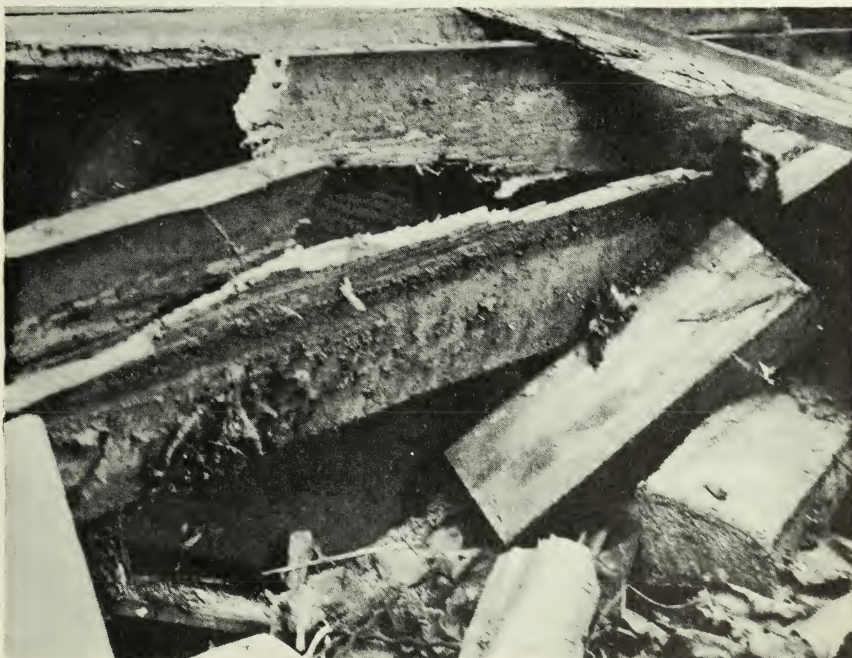
Figure 4. - Collapsed post and broken sheathing, 60-year old house, Victoria, B.C.
