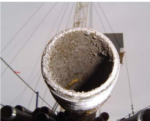
Pipeline contaminated with NORM (Photo courtesy of Tervita Corporation)
