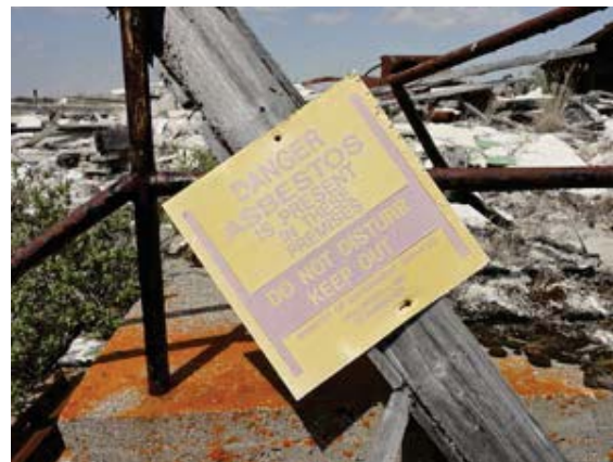
Signage at a Mid-Canada Line site warns of demolition debris from a collapsed building containing asbestos.
