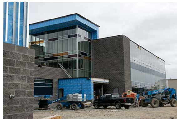
The new Transport, Electrical, and Mechanical Engineering (TEME) facility at CFB Halifax is the new home of TEME operations at the base. The 12,000-m 2 , two-storey building accommodates dispatch functions, administration, shops and training facilities.
