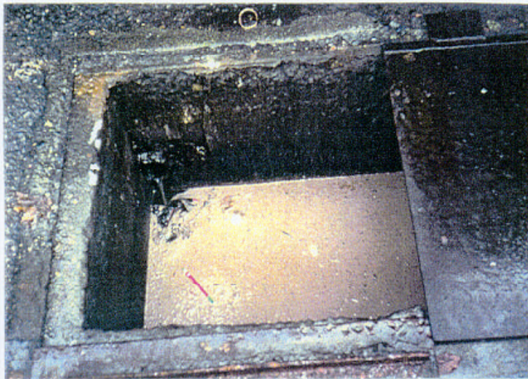
CHAMBER 1 AND OUTLET FROM WASH BAYS 4, 5, 6
