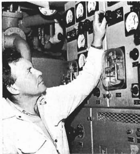
Chief engineer on board the YBZ-61 is Percy Carr, shown at work on one of the control panels in the cleansing barge. Working with Mr. Carr is a crew of four men, made up of two oilers and two firemen. (G-74890)
