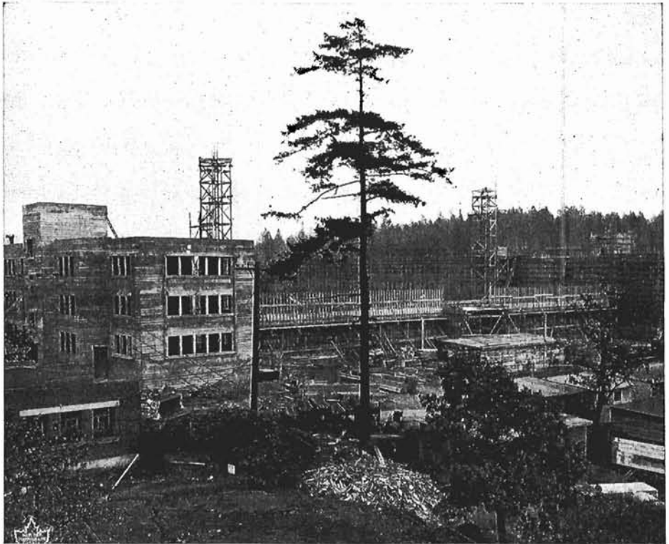
Among the more ambitious construction projects undertaken by the Royal Canadian Navy in 1952 was the new barracks block at HMCS Naden. Construction was started last January and the above picture shows progress toward the end of the year. (E-20834).
