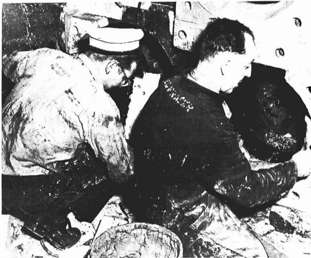
Happy although the lot of the man in the boiler room may be today compared with his existence in the coal-burning era, there are still a few important jobs which are a bit on the messy side. This picture is of brickwork being repaired in HMCS "Huron's" No. 3 boiler during her first tour of duty in the Far East. (HU-75)
