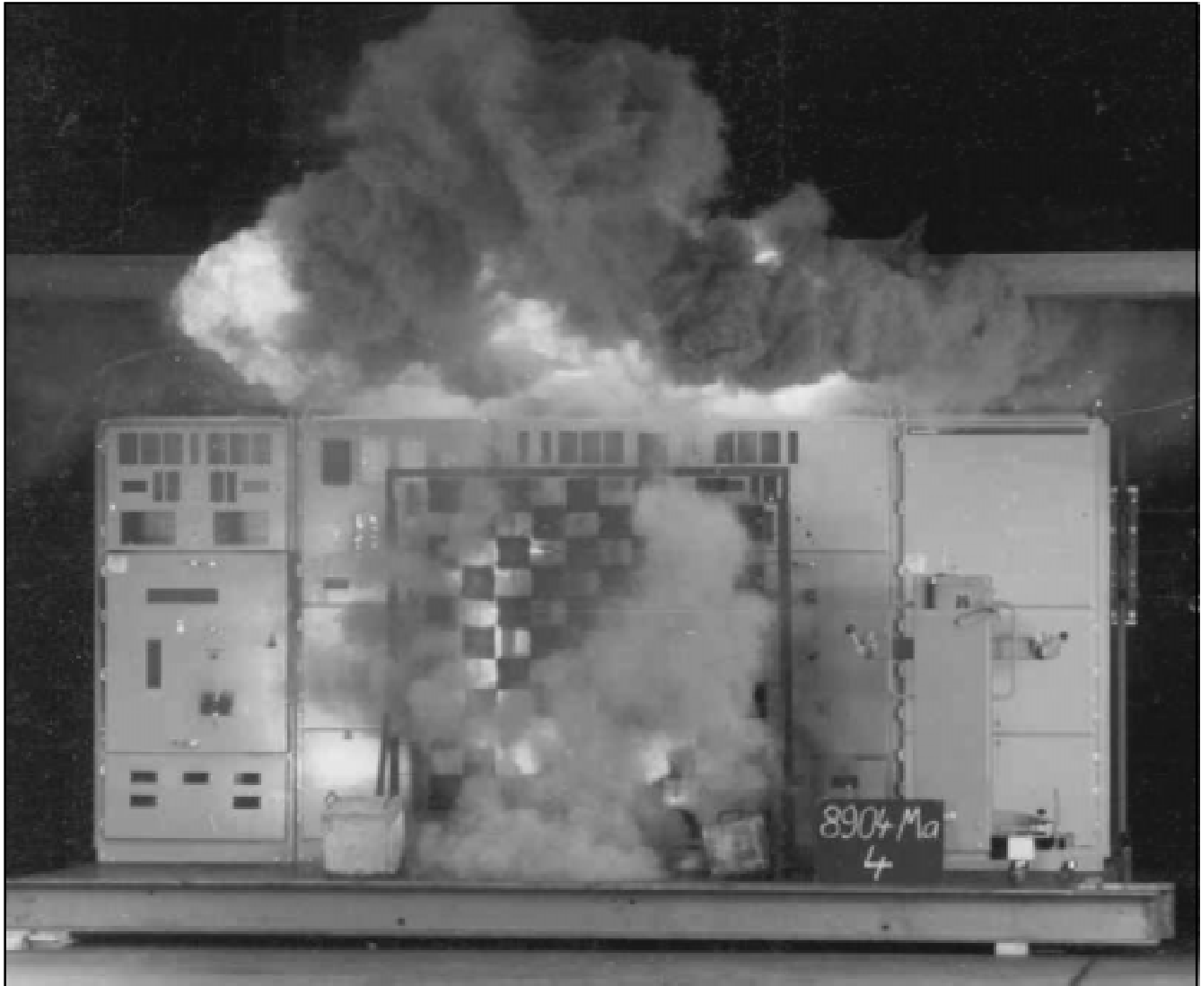
Fig. 1. This dramatic test bay photo was taken approximately 0.9 seconds after a short-circuit was ignited in a medium-voltage breaker compartment running 15-kV, 40-kA, 1-second arc-resistant metal-clad switchgear. Pressure release flaps on the top of the compartment opened to release hot by-products of the short-circuit explosion before the rising pressure could blow the doors and bolt-on panels on the front of the compartment open. In a real situation, this action would have prevented injury to personnel standing in front of the breaker compartment. (Courtesy Siemens Canada Ltd.)
