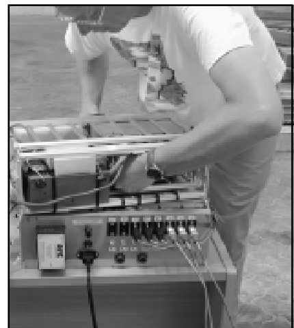
Kevin Ferguson (top) splices a sensor cable damaged by coral, while Phil Thornton (middle) makes soldering repairs. Kevin Ferguson connects up the signal amplifiers (bottom).
