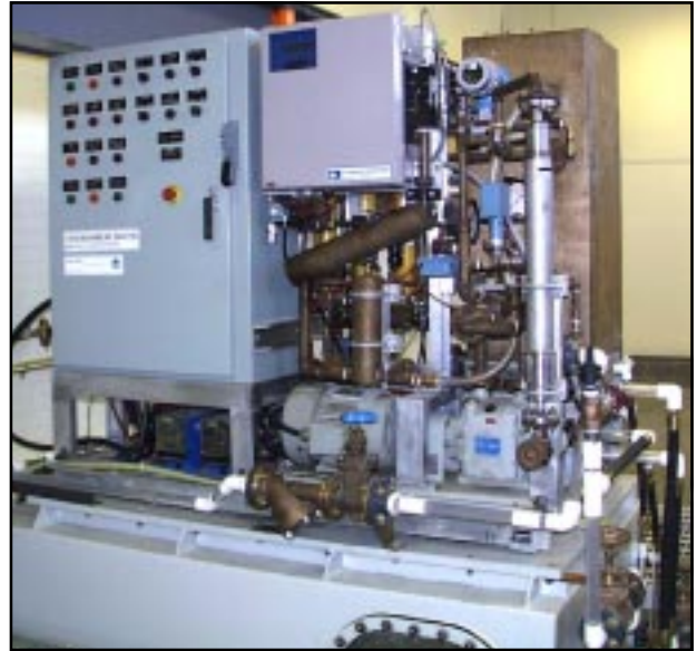
This working Hydromem unit is installed at the Canadian Forces Naval Engineering School in Halifax to support QL5 Mar Eng Tech training.
