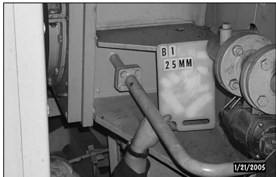
Fig. 3. The oil supply line to bearing no. 1 is nearly one metre long, but is supported only by a very small weld where it enters the gearbox casing. The presence of a flanged connection within a few centimetres of the weld point could be adding stress to the weld if the flange connection itself is under stress. As can be seen, the oil line provides a convenient, but damaging foothold for personnel climbing up to the casing top.
