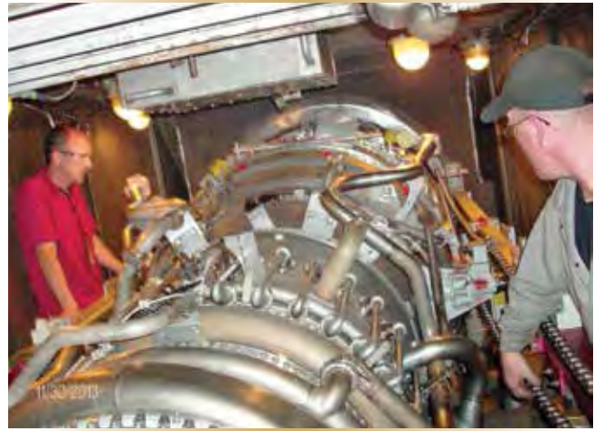
Figure 13 – GE field service rep Del Rogers (left) and FMFCS navy GT tech LS John Alford mate the gas generator to the power turbine. The ship went on to conduct sea trials days ahead of schedule.
