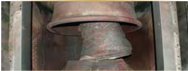
Figure 4 – Looking down into the engine exhaust duct of the enclosure, ship's staff get their first view of the damage to the HSCS.
