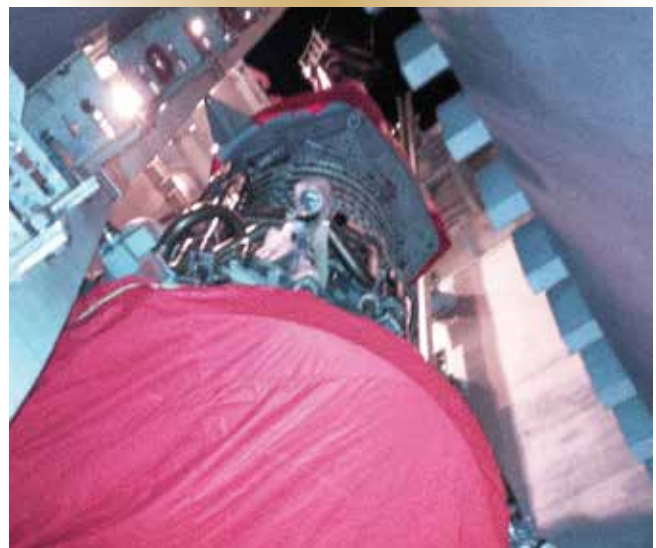
Figure 7 – Up and out. The gas generator is hoisted up the air intake by shore crane.
