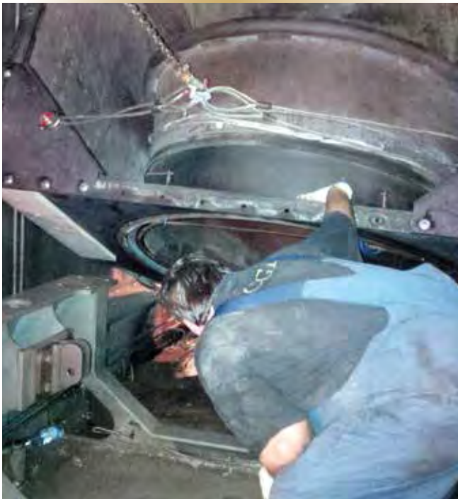
Figure 8 – FMFCS rigger Steve Eddy guides the exhaust duct into a horizontal position.
