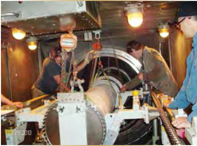
Figure 12 – FMFCS rigger Joshua Gordon, plater Ricardo Green and HMCS Toronto 's PO1 Steve Beaulieu install the new high-speed coupling shaft.
