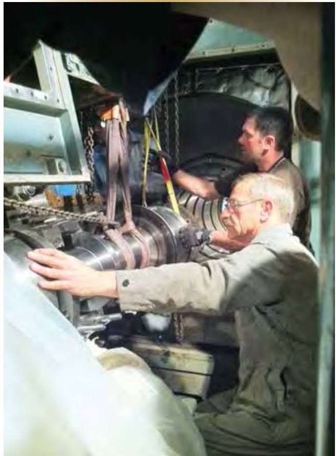
Figure 11 – Things begin to come together. With the new exhaust duct in position, the author (foreground) and FMFCS rigger Spartius Toope can install the replacement GT input shaft.
