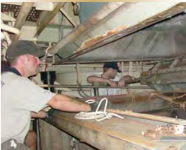
Figure 6 – With the exhaust expansion joint moved forward, FMFCS rigger Spartius Toope (left) and plater Ryan Shaw have cleared the way for the exhaust duct to be rotated into position for removal.
