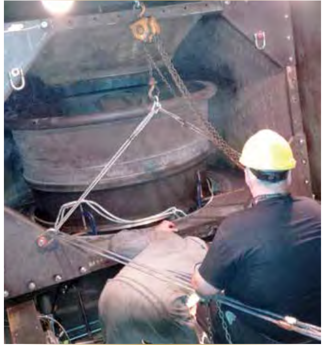
Figure 9 – Clearances were as little as 3 mm as the exhaust duct was moved carefully through the enclosure for removal.
