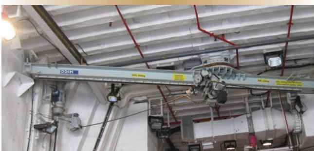
Figure 1. The MHP crane as fitted in HMCS Montréal 's hangar. The ship was the designated frigate for the Maritime Helicopter Project acceptance trials.
