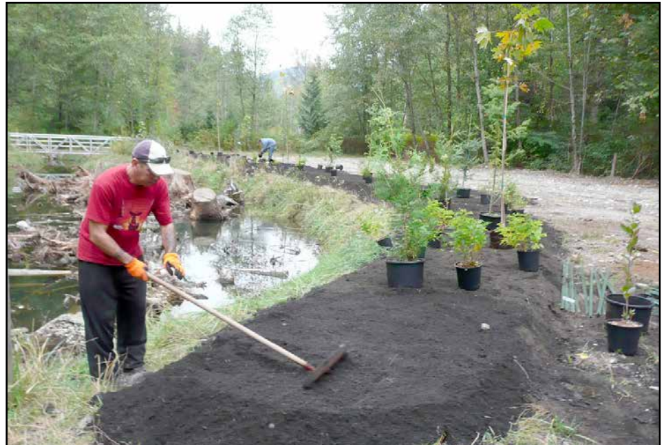
The gravel stockpile, rocks, and roots at Oxbow Pond were removed. Then 25 metres of topsoil were imported and planted with shrubs and trees to help stabilize the bank and provide shade. Photo: Watershed Watch Salmon Society.
