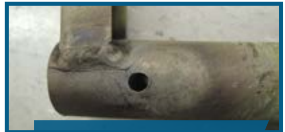
Bolt Hole Crack
