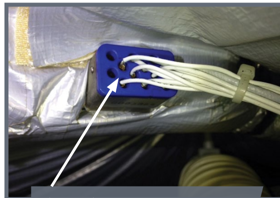
Wiring fault causing an intermittent failure of the flight data recording system
