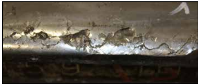
Photo 6. Shelling on the gauge face of the rail
