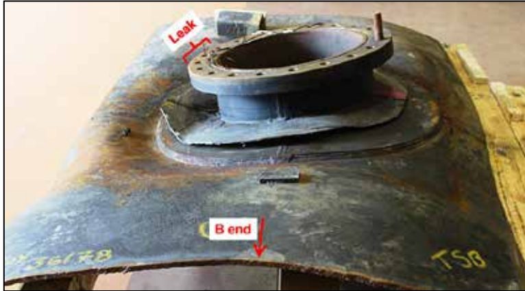
Figure 5. Photograph taken after removing the tank jacket to expose the weld joining the manway nozzle reinforcement to the tank. Note tank deformation near the leak location.
