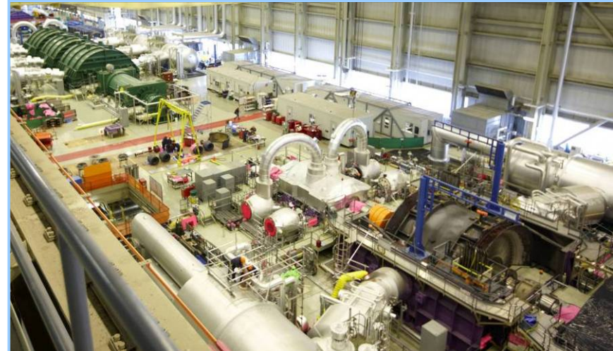
Darlington Nuclear Generating Station (turbine hall), Clarington, ON
