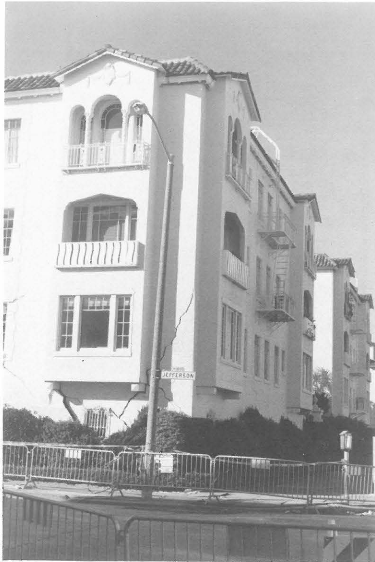
Fig. 2.5 House damaged by differential settlement due to soil liquefaction in Marina District, San Francisco
