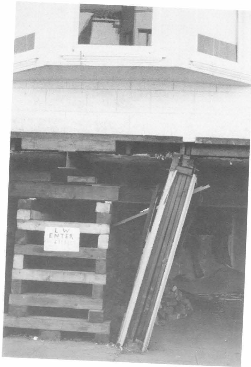
Fig. 3.14. Inadequate connection detail between post and floor framing in the corner 4-storey apartment building in Marina District, San Francisco
