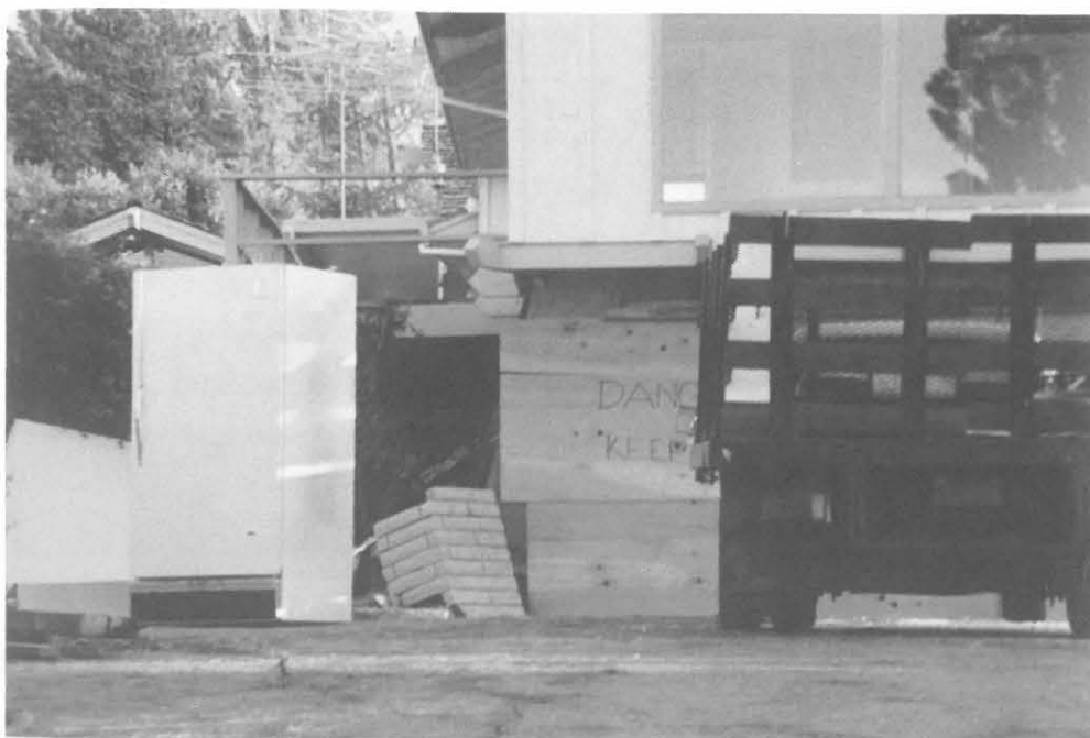
Fig. 3.9 Lack of lateral resistance and creation of two hinges in garage posts contributed to damage (note destroyed brick veneer wall)
