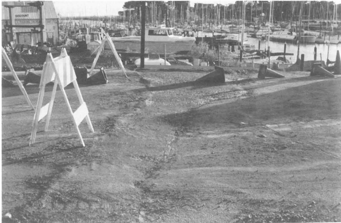
Fig. 4.26 Filled fissure which caused a break of the water pipe - bridge on Eaton Street in Santa Cruz
