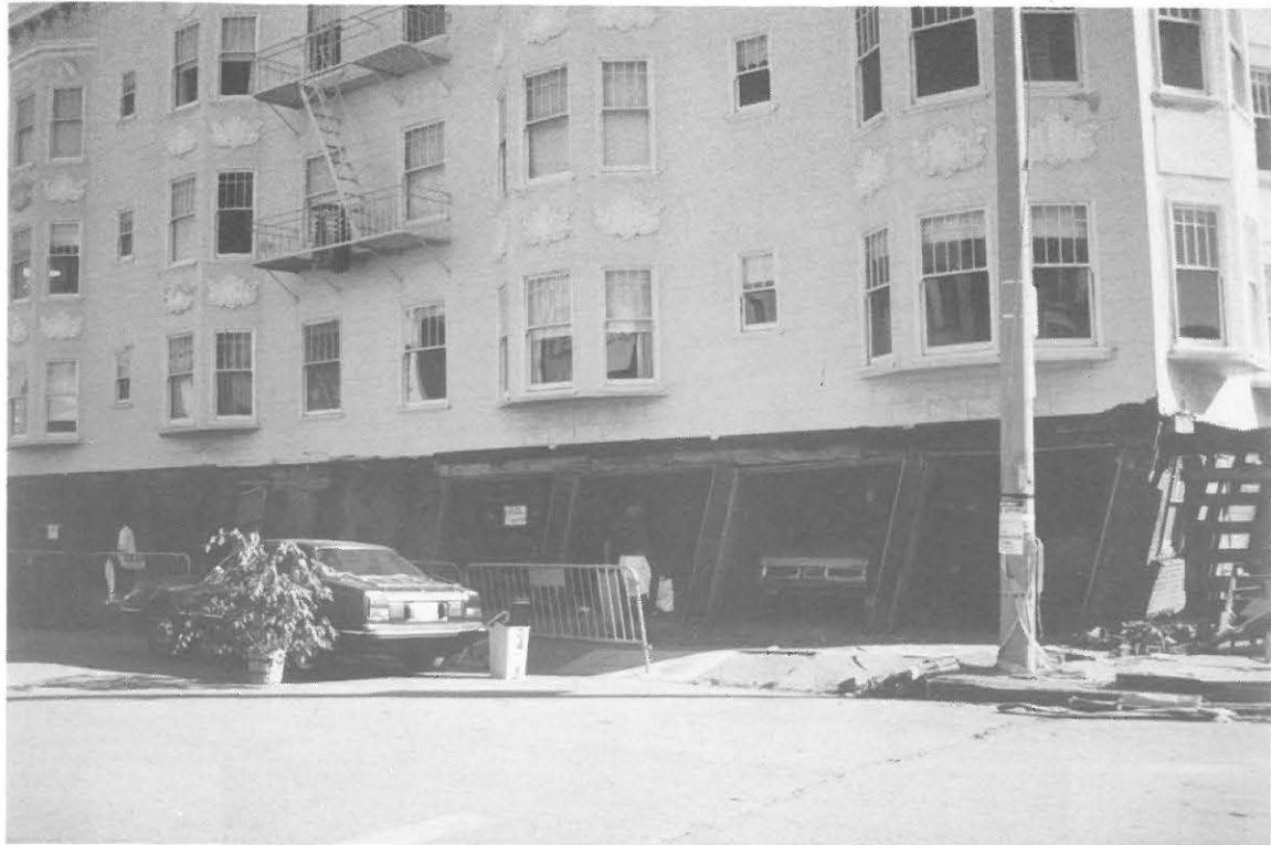
Fig. 3.13. Another example of "soft storey" effect on Jefferson St., Marina District, San Francisco (note horizontal boards on posts and over the garage doors)
