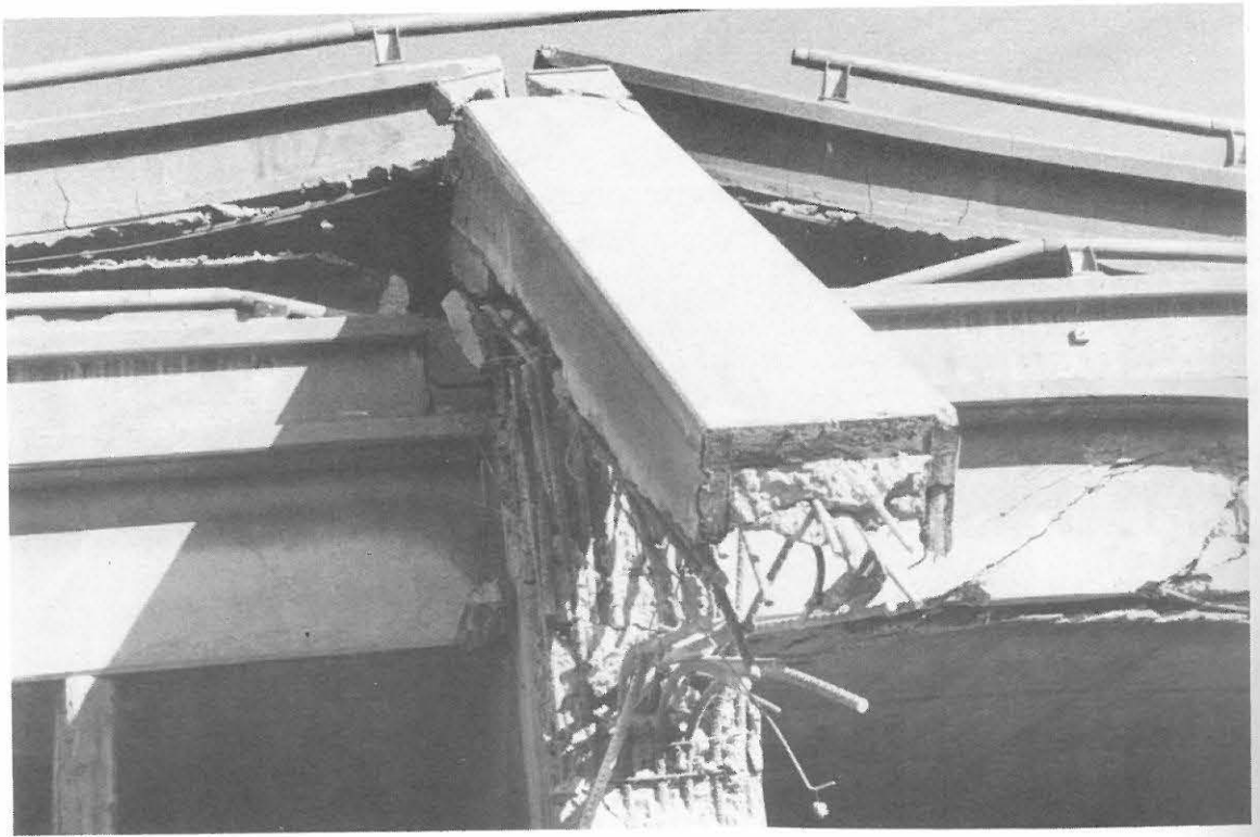
Fig. 4.5 Detail of upper column failure
