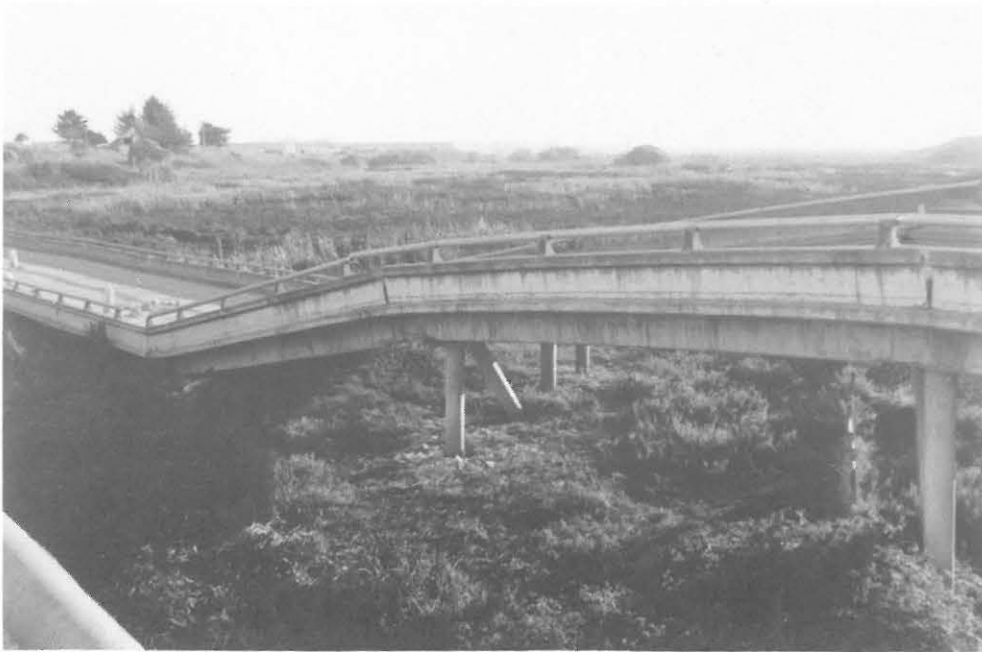
Fig. 4.17 The difference between levels before and after collapse - the Struve Slough Bridge
