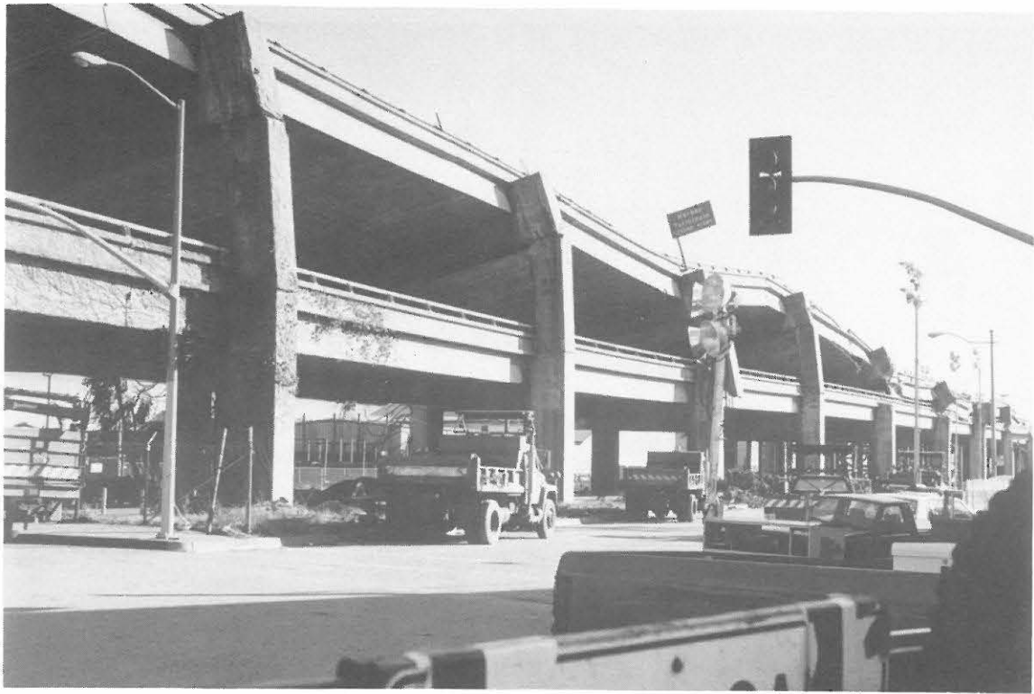
Fig. 4.7 Partial collapse of upper deck
