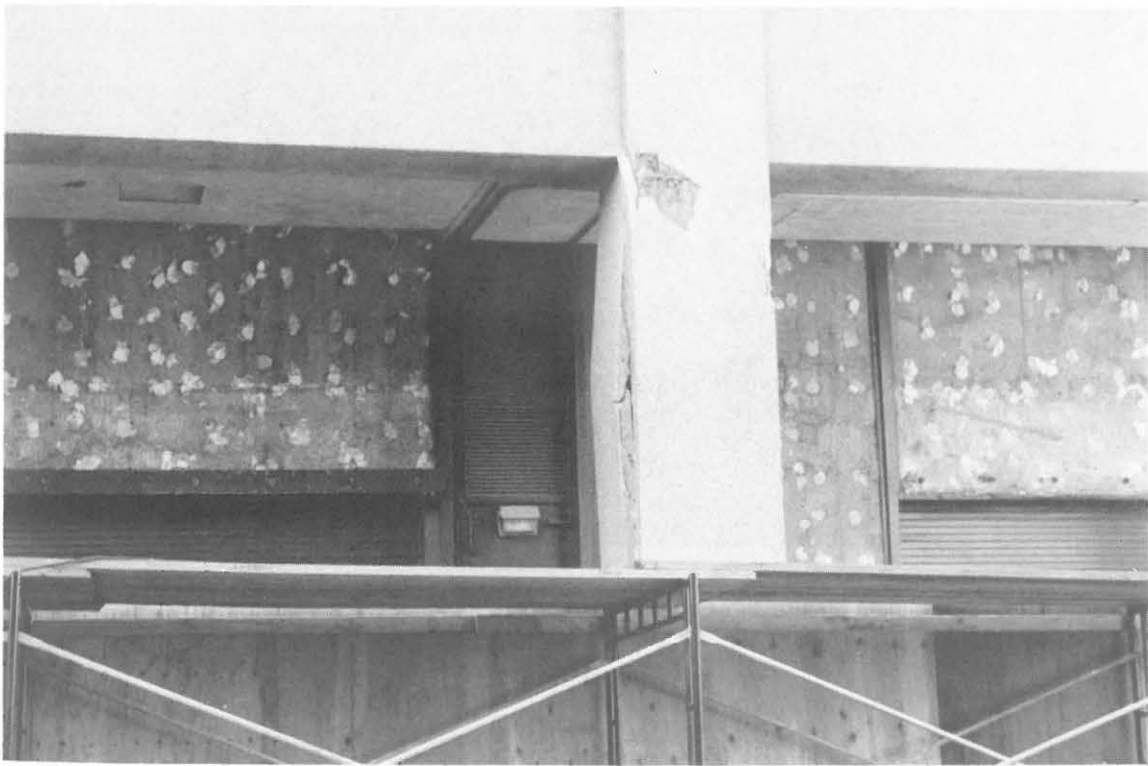
Fig. 3.22. Damage to column in high-rise building in downtown Oakland
