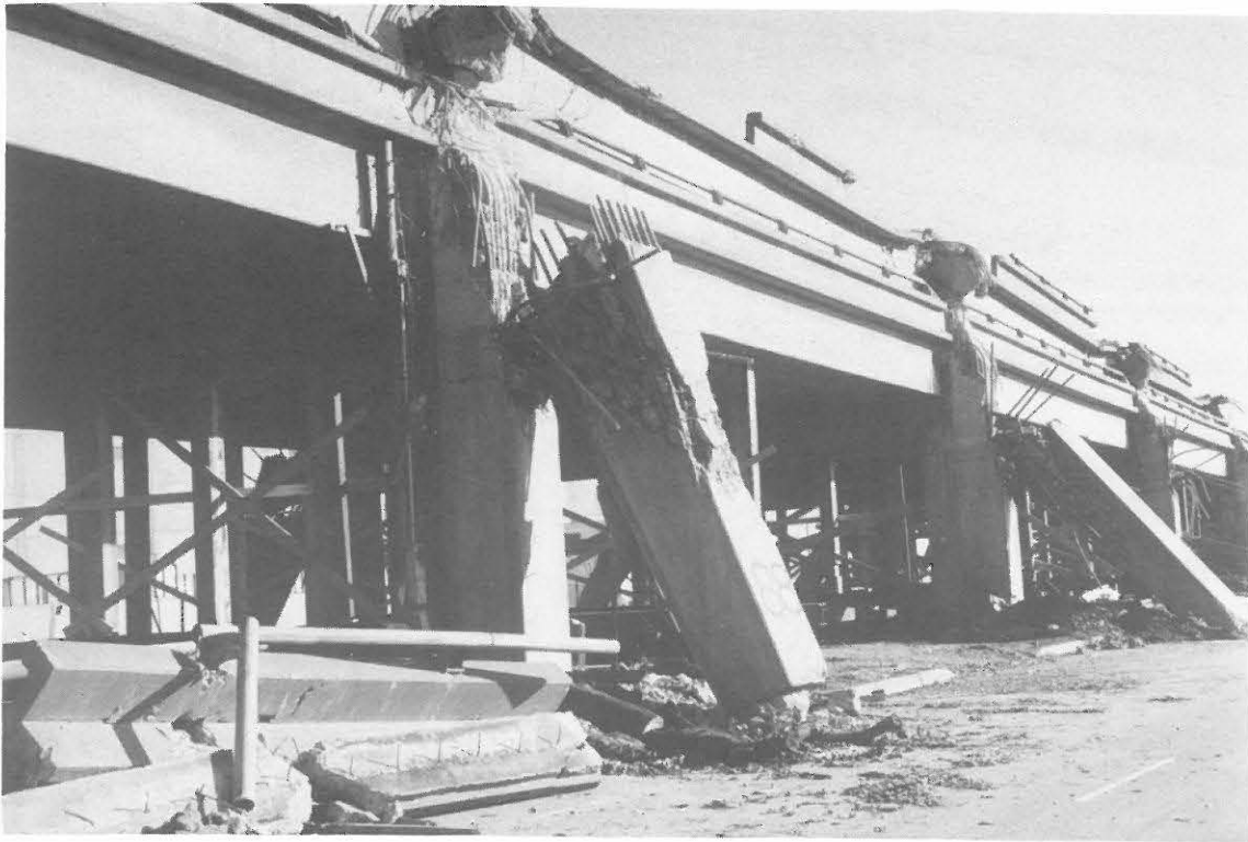
Fig. 4.3 Collapsed Cypress Street viaduct
