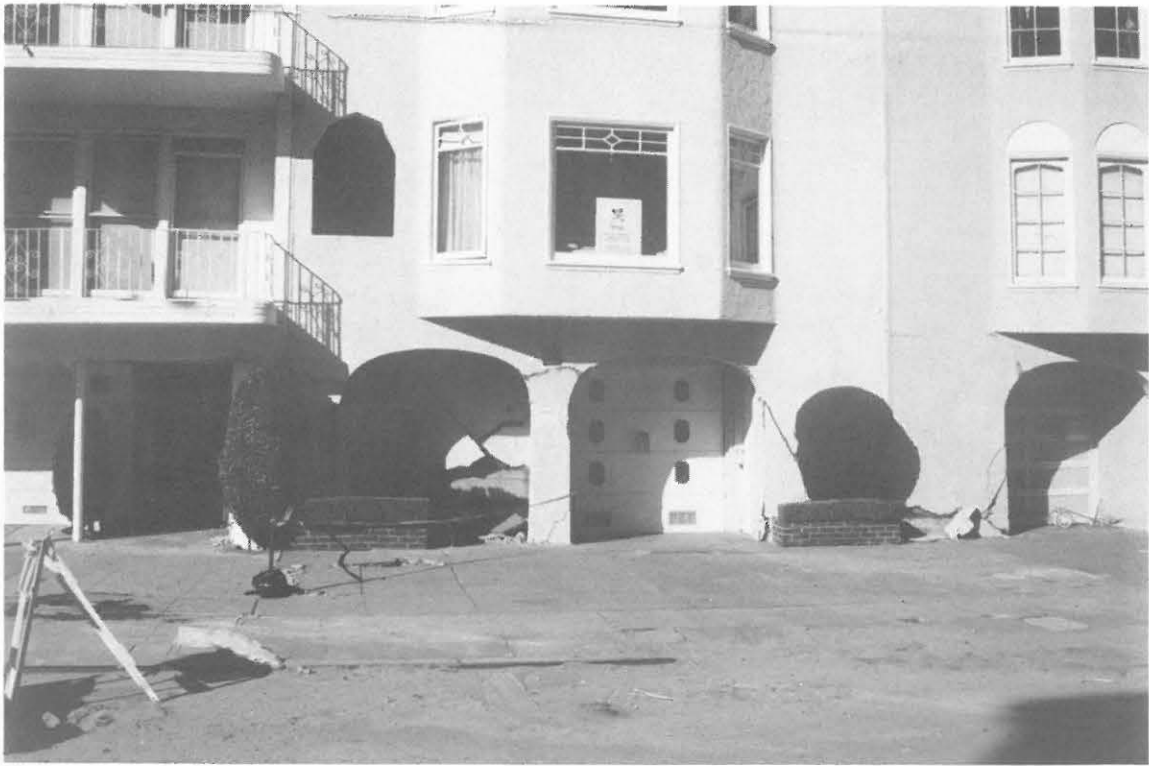
Fig. 3.17. An example of 3-storey building covered with stucco which experienced minor damage over openings at the first floor level - Marina District, San Francisco
