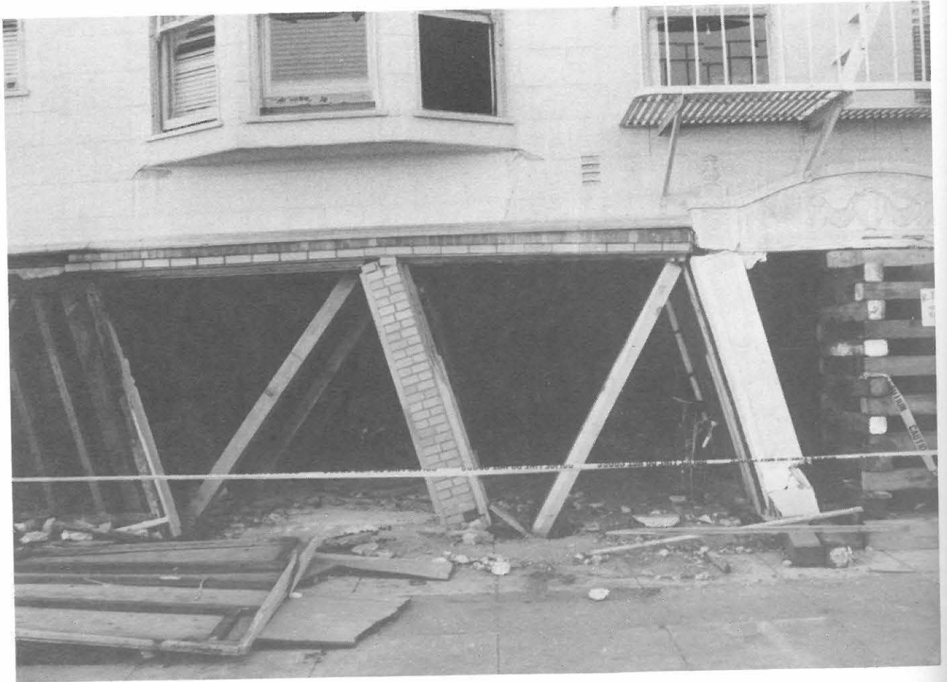
Fig. 3.12. Close-up of the first "soft storey", Beach/Broderick Streets, Marina District, San Francisco
