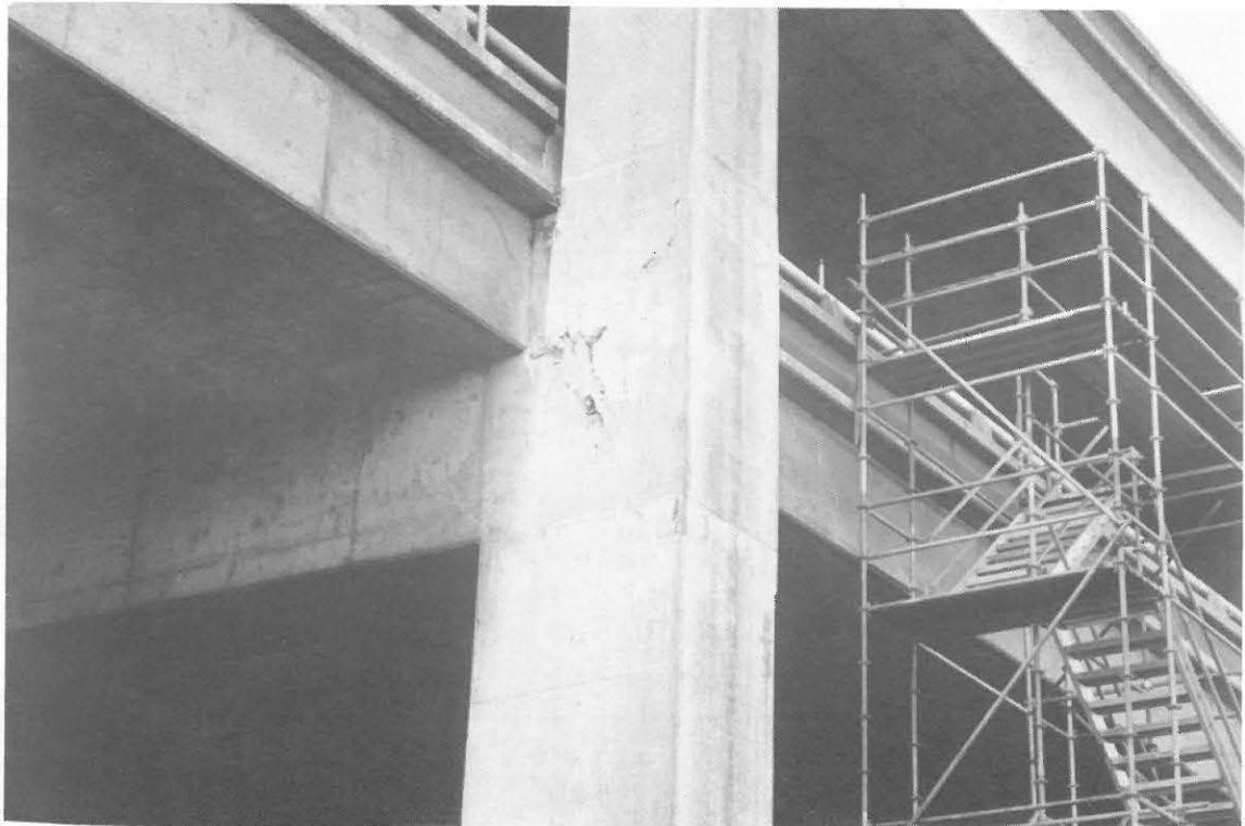
Fig. 4.8 Diagonal shear cracks in Embarcadero Freeway
