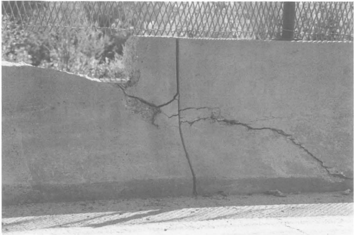
Fig. 4.21 A destroyed road barrier on Highway 17 near Los Gatos
