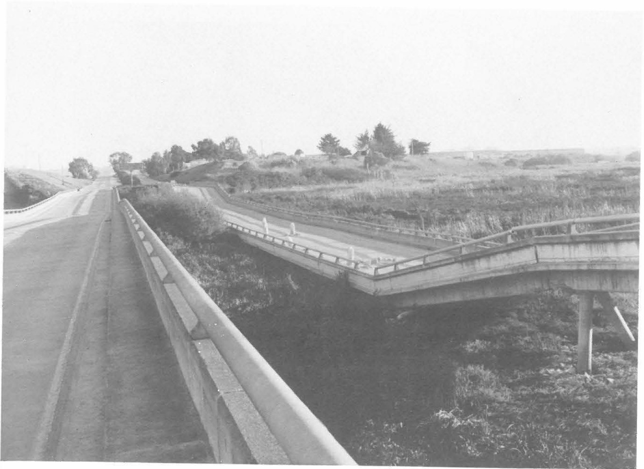
Fig. 4.14 The two heavily damaged lanes of the Struve Slough Bridge on Highway 1 near Watsonville
