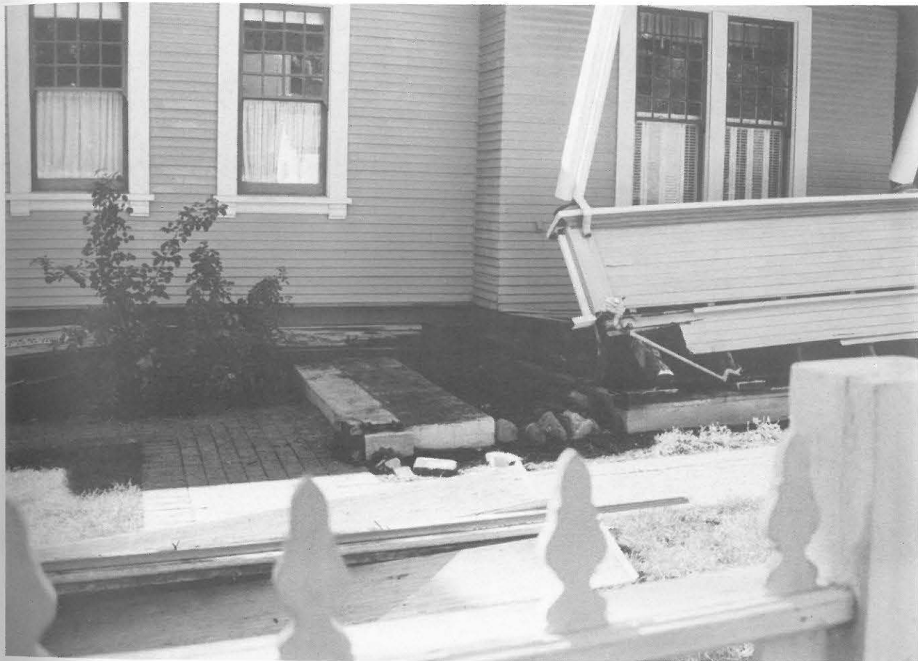
Fig. 3.6 House shifted from the foundation by approximately 18" (45 cm) and the small staircase to the porch destroyed and removed in a residence on Main Street in Los Gatos
