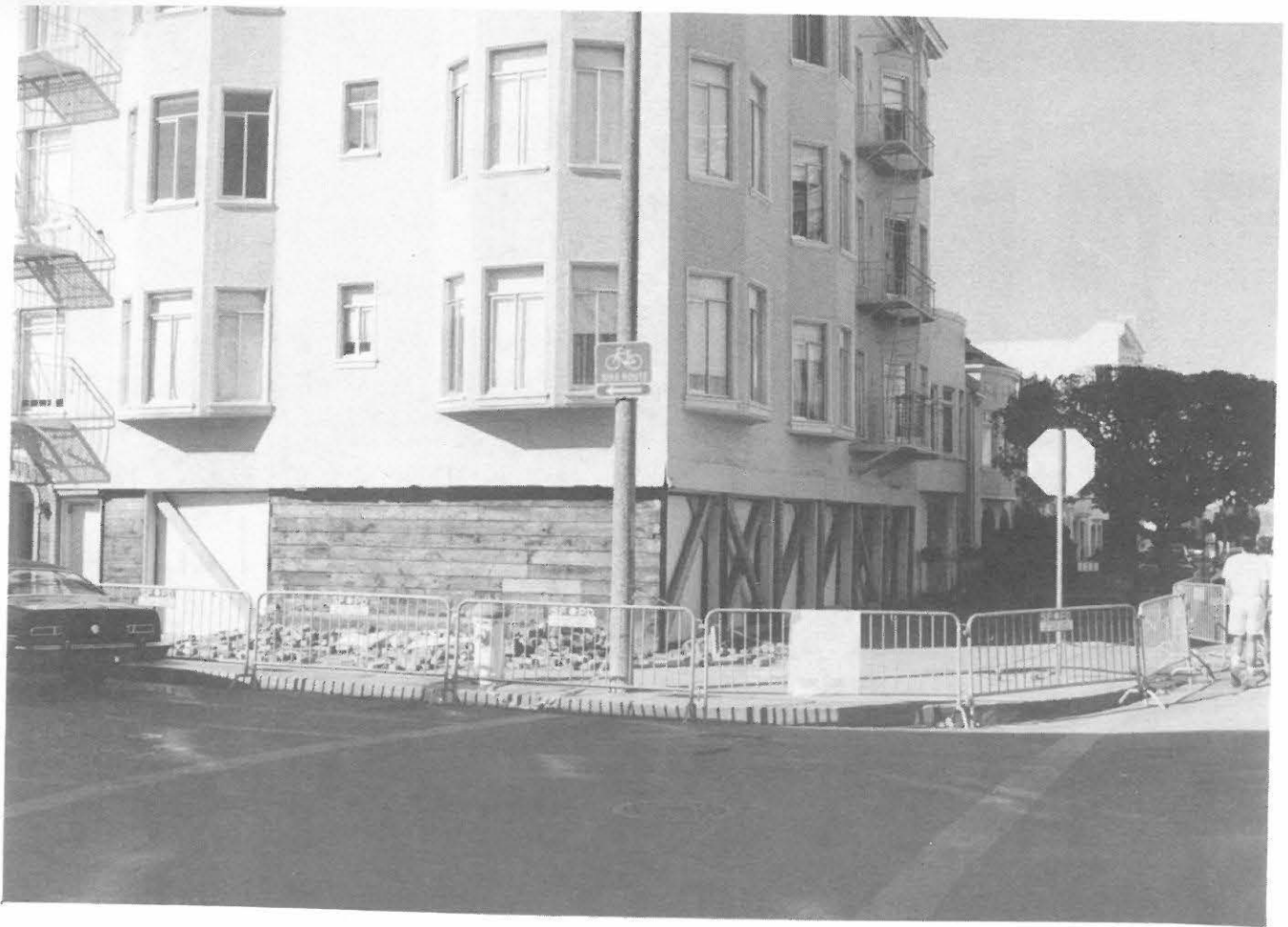
Fig. 3.16. 4-storey apartment building with destroyed brick wall - Marina District, San Francisco
