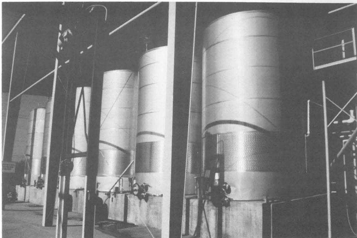
Fig. 6.3 The outdoor stainless steel tanks with cooling jackets
