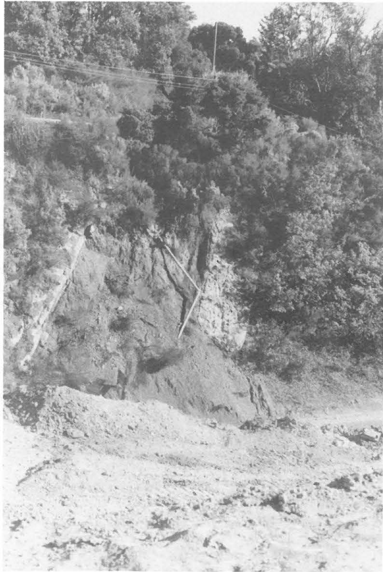
Fig. 2.8 Landslide on Highway 17
