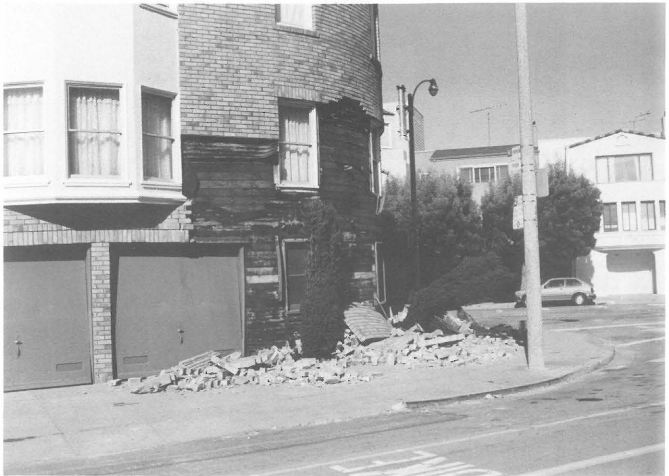
Fig. 3.15. 4-storey apartment building with more sheathed walls (horizontal boards) experienced less damage and much less horizontal shift - Marina District, San Francisco
