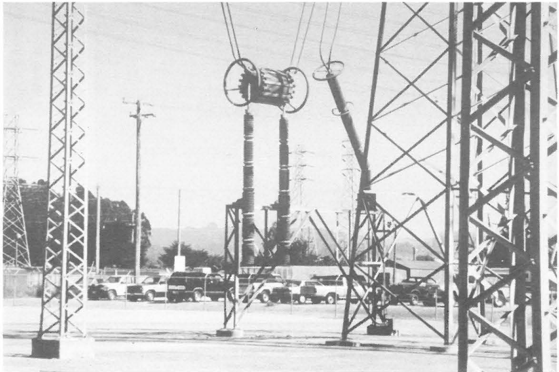
Fig. 5.12 Damaged 500-kV tension transformers at Moss Landing (courtesy of J.W. Lafferty, PG&E)
