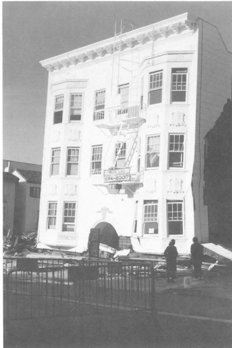
Fig. 3.10. A 4-storey wood-frame multi-apartment house reduced to 3-storey building in the Marina District, San Francisco
