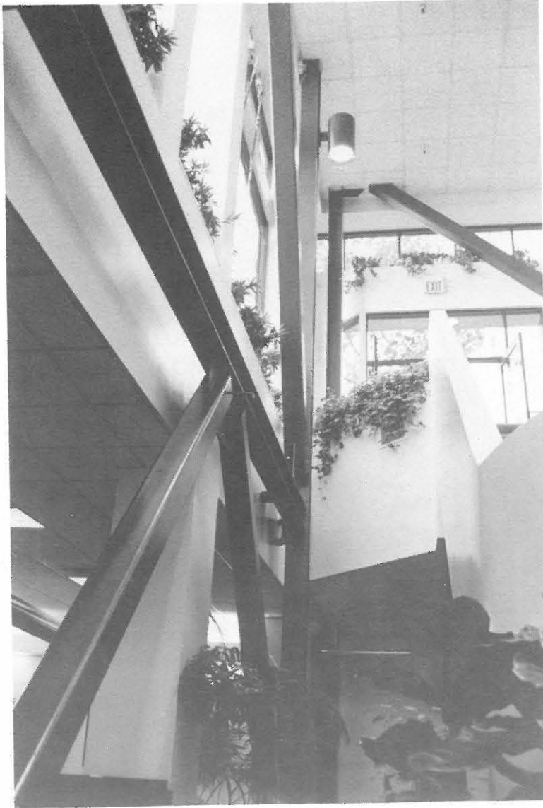
Fig. 3.25. An old structure of the corner building upgraded after 1971 San Fernando earthquake performed well
