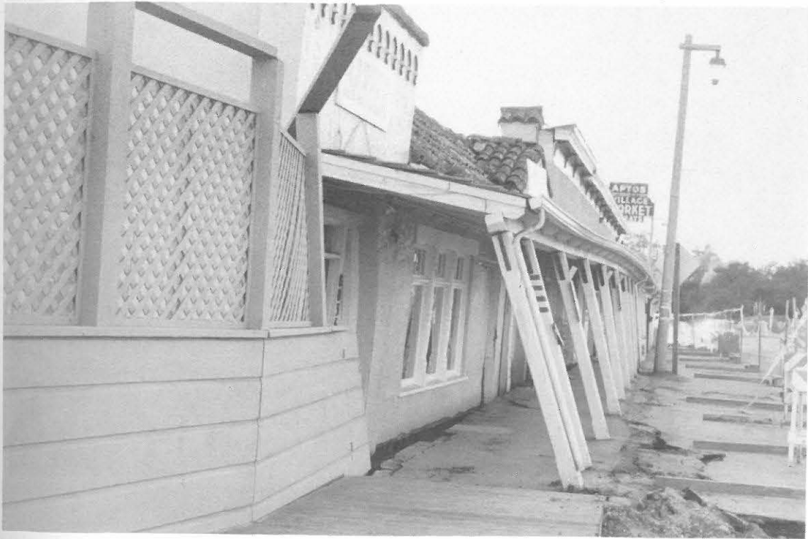
Fig. 2.3 Partially collapsed house due to liquefaction failure in Aptos, 9.5 km from epicenter
