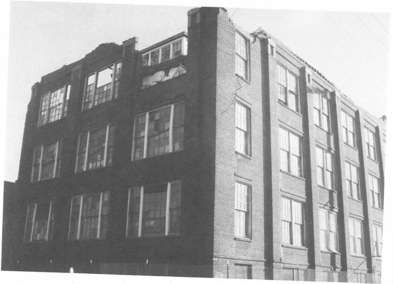
Fig. 3.20. A 4-storey storage building on Campbell Street in Oakland with damage to the parapet walls and collapsed roof
