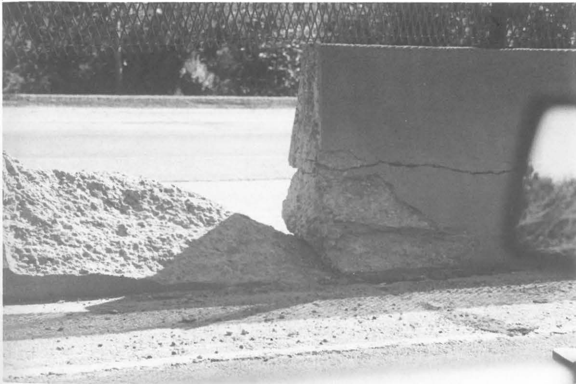
Fig. 4.22 A large horizontal displacement caused damage to the road barriers on Highway 17
