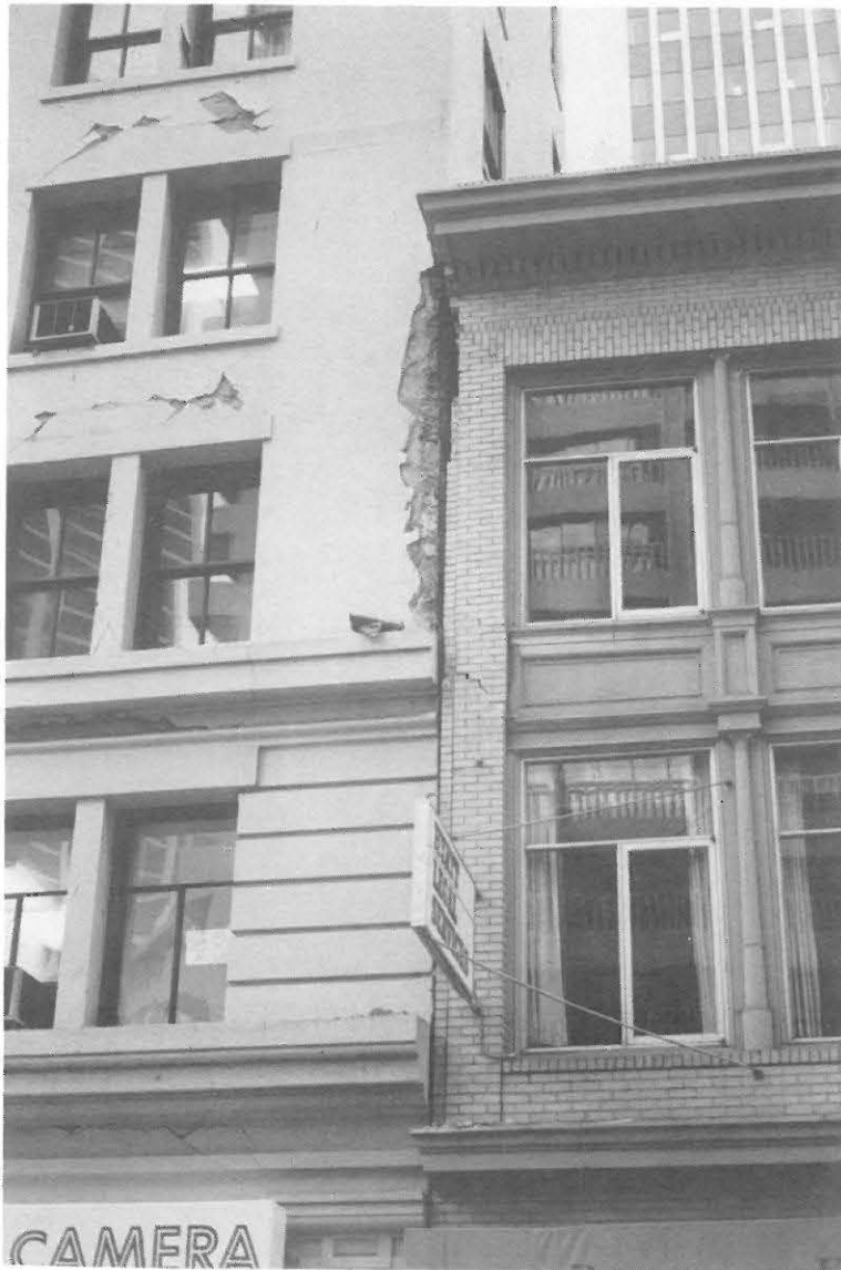
Fig. 3.23. An example of pounding between two adjacent buildings, Mission Street, San Francisco
