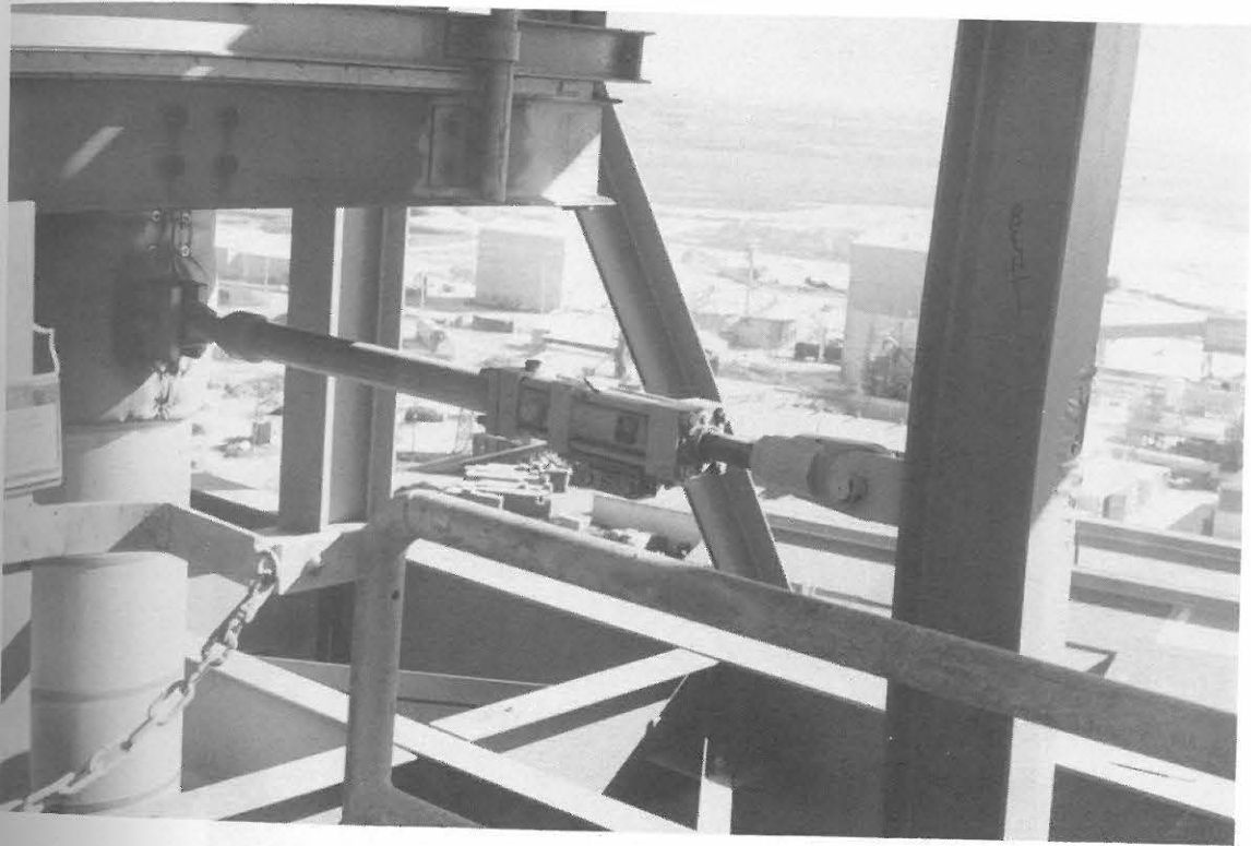
Fig. 5.4 Damage to a vertical strut supporting a horizontal snubber
