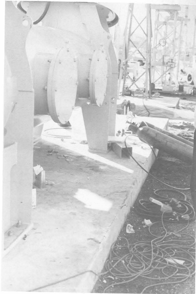
Fig. 5.33 New circuit breaker support
