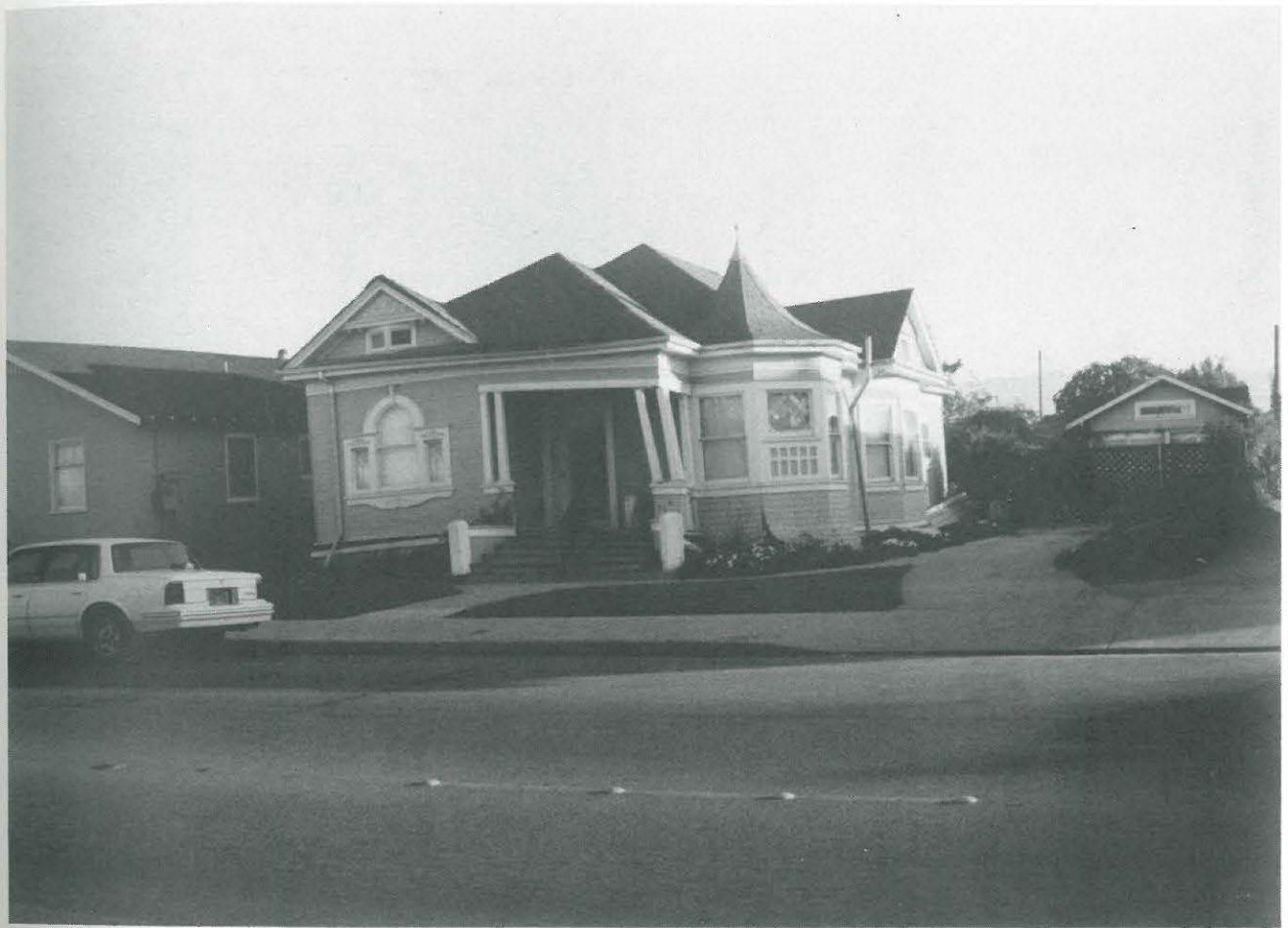
Fig. 3.1 An old residence with cripple wall failure affecting integrity - 114 Brennan Street in Watsonville
