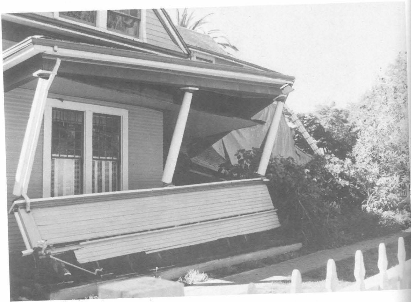
Fig. 3.5 Collapsed cripple wall and porch in an old residence at Main Street in Los Gatos
