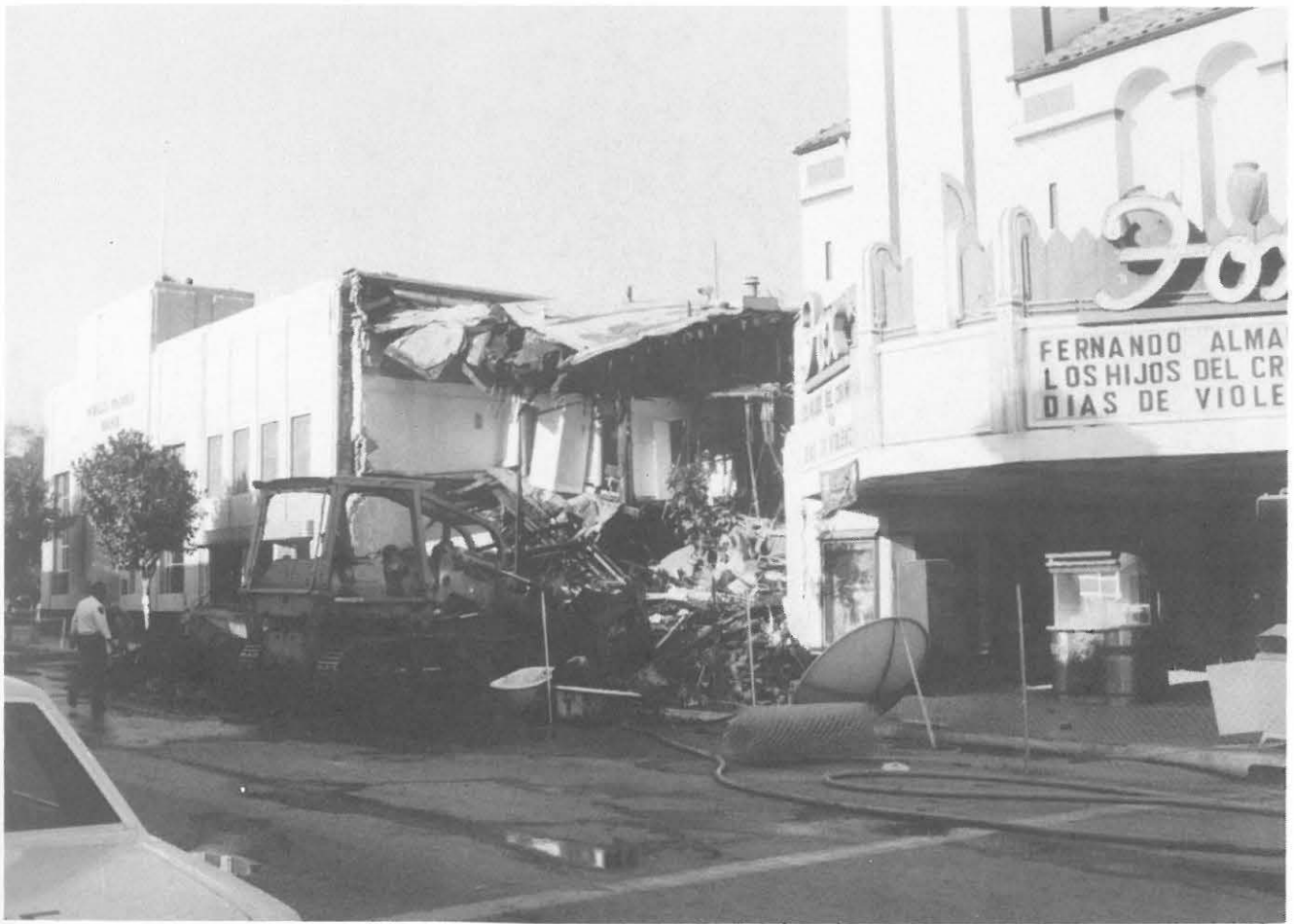
Fig. 3.19. Demolishing process of the heavily damaged unreinforced masonry building on Main Street in downtown Watsonville
