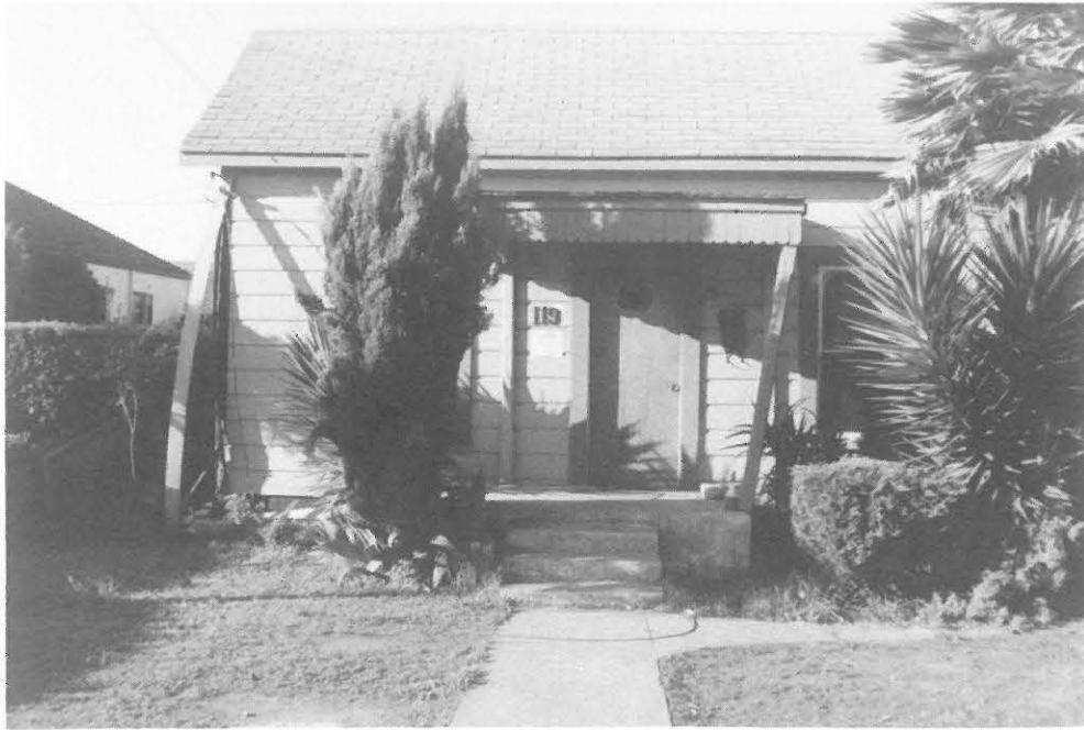
Fig. 3.3 The collapsed cripple wall shifted this house by more than 1' (32 cm) at 119 Sudden Street in Watsonville
