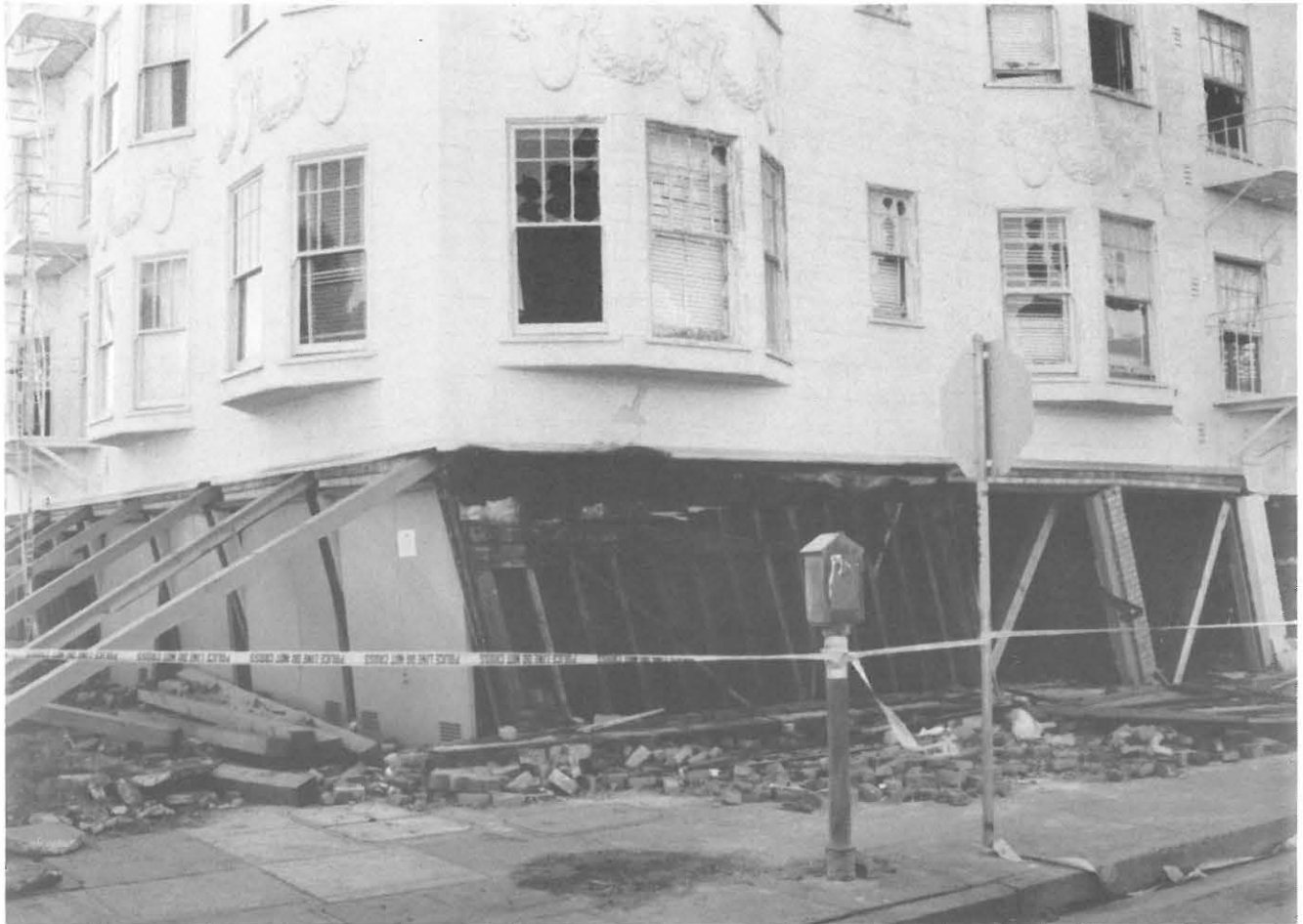
Fig. 3.11. Almost collapsed 4-storey wood-frame apartment building due to "soft storey" effect at the corner of Beach and Broderick, Marina District, San Francisco
