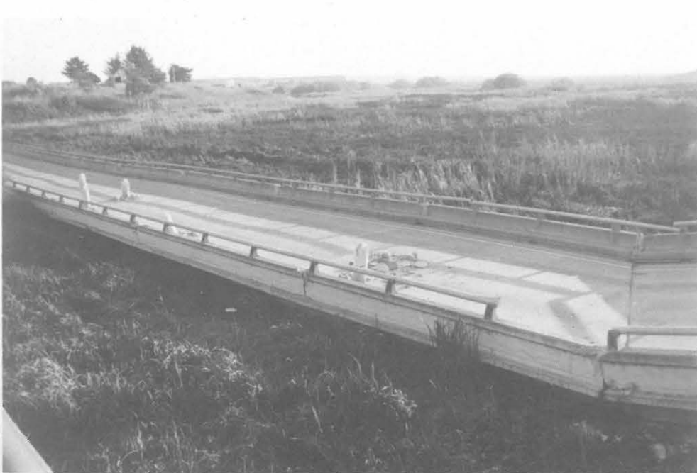
Fig. 4.18 The collapsed portion of the deck of the Struve Slough Bridge did not disintegrate during the earthquake
