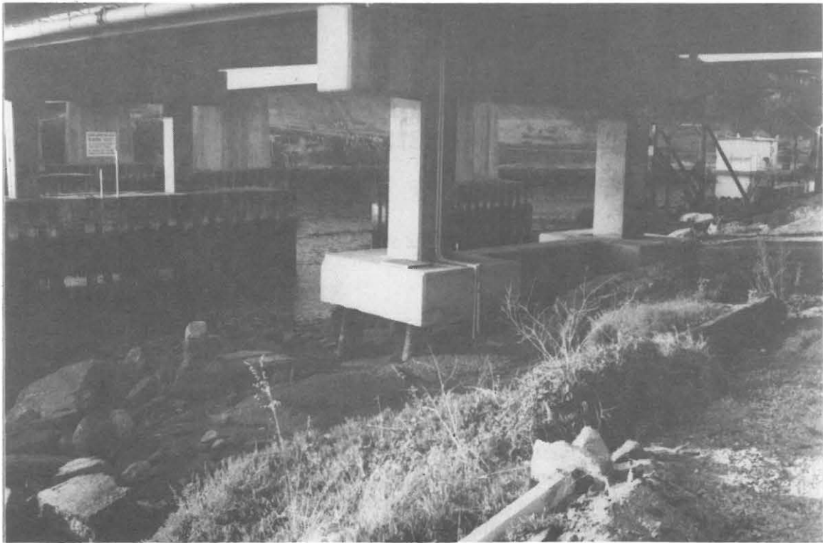
Fig. 4.25 Water from a broken pipe caused damage to the pier of the bridge on Eaton Street in Santa Cruz
