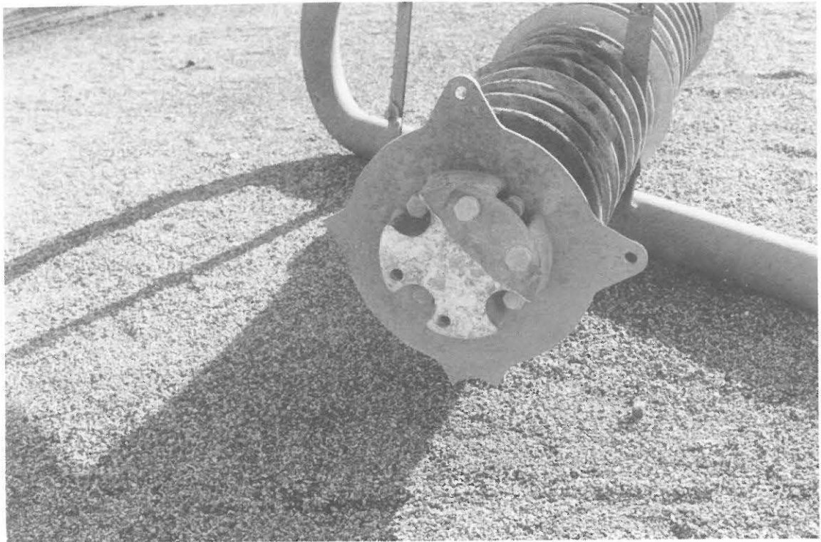
Fig. 5.18 Remains of a destroyed 500-kV disconnector. Failure of a flanged cap
