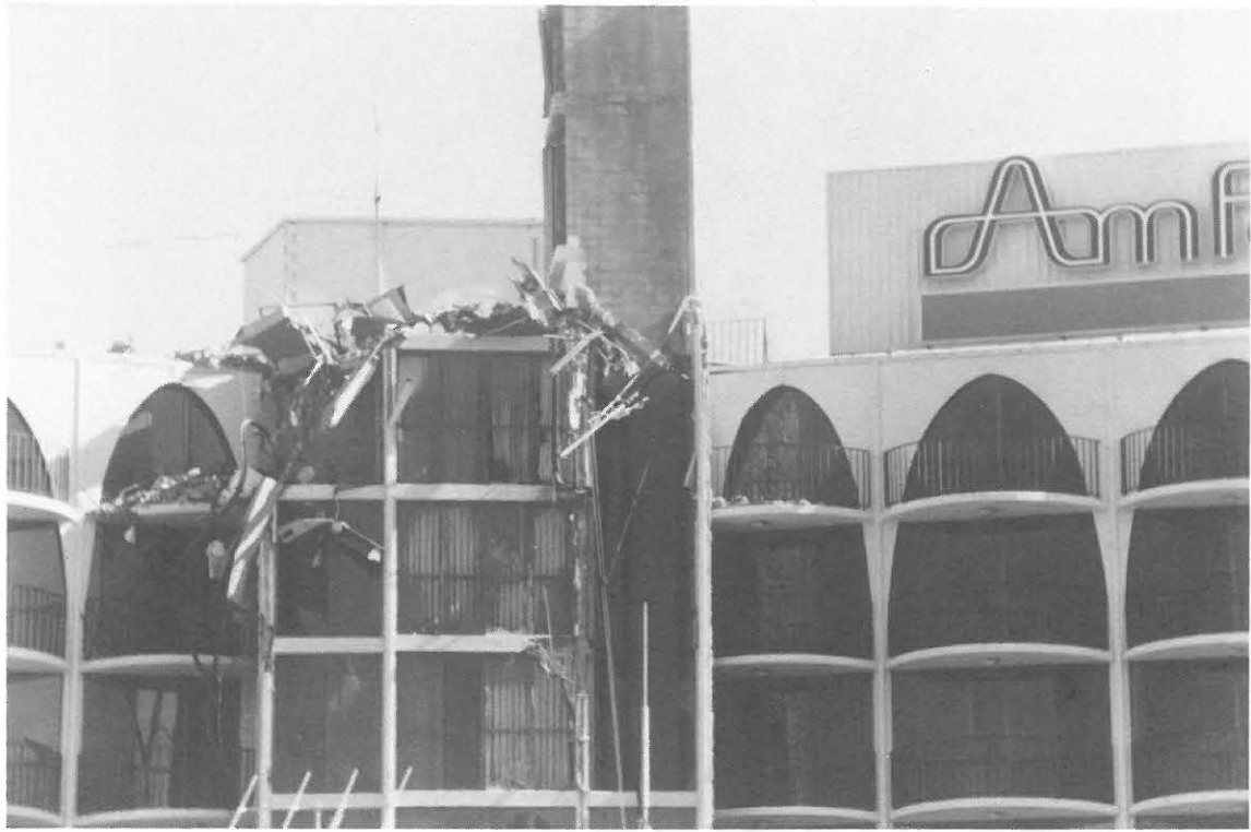
Fig. 3.24. Collapsing water tank destroyed a penthouse at the top of Amfac Hotel at the San Francisco Airport
