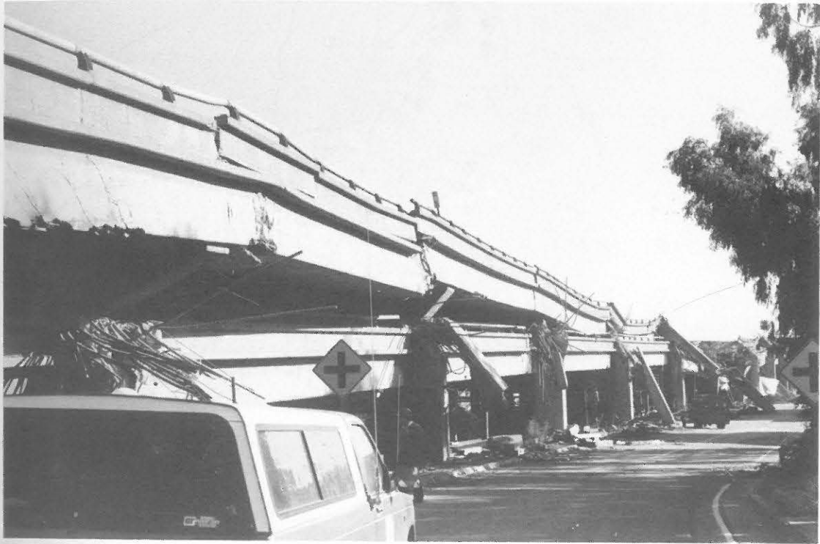
Fig. 2.1 The collapse of the Nimitz Freeway in Oakland
