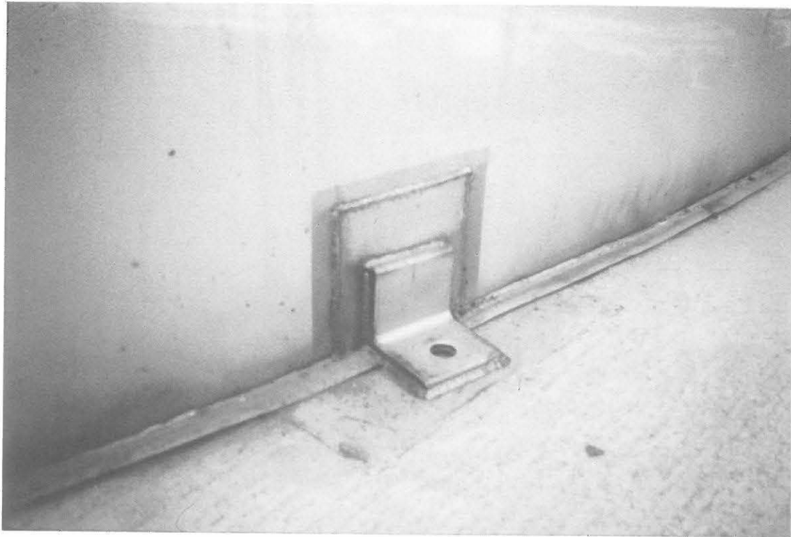
Fig. 6.15 Anchorage of undamaged tank
