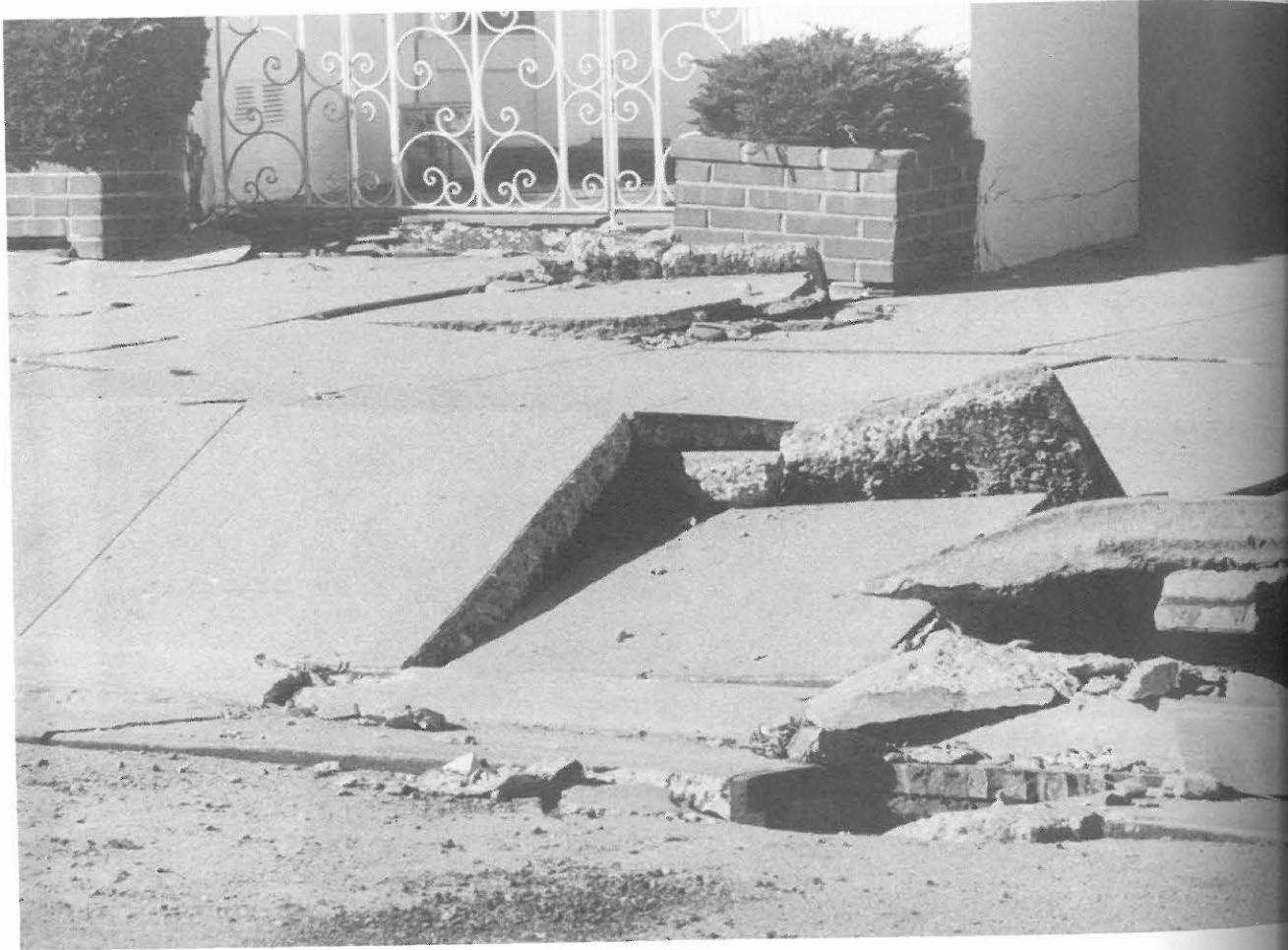
Fig. 2.6 Buckled sidewalk due to soil liquefaction in Marina District
