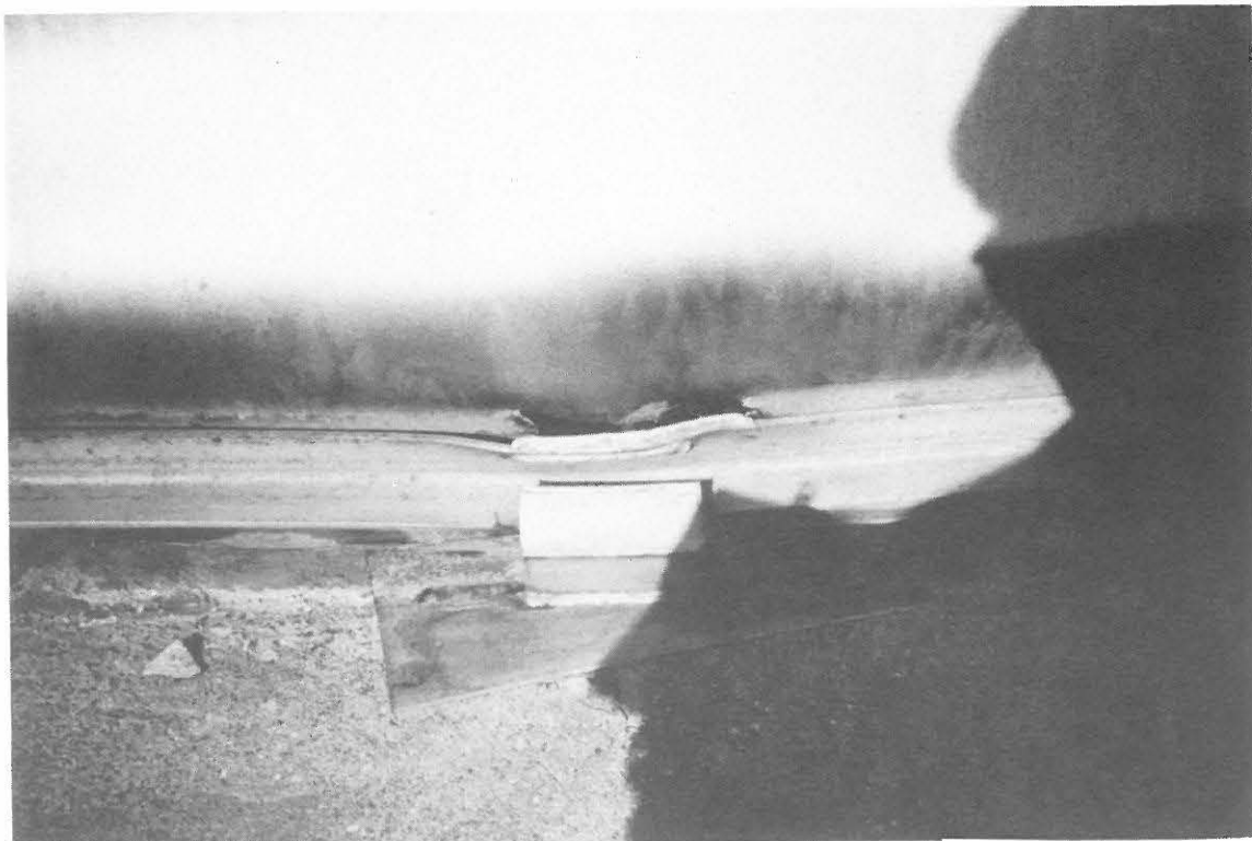
Fig. 6.14 Failure of welded angle plate
