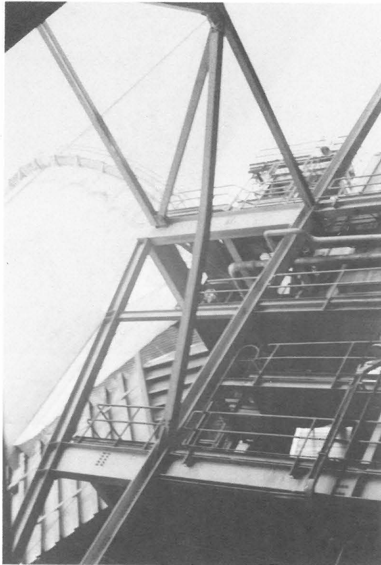
Fig. 5.3 Damage to two bracing members
