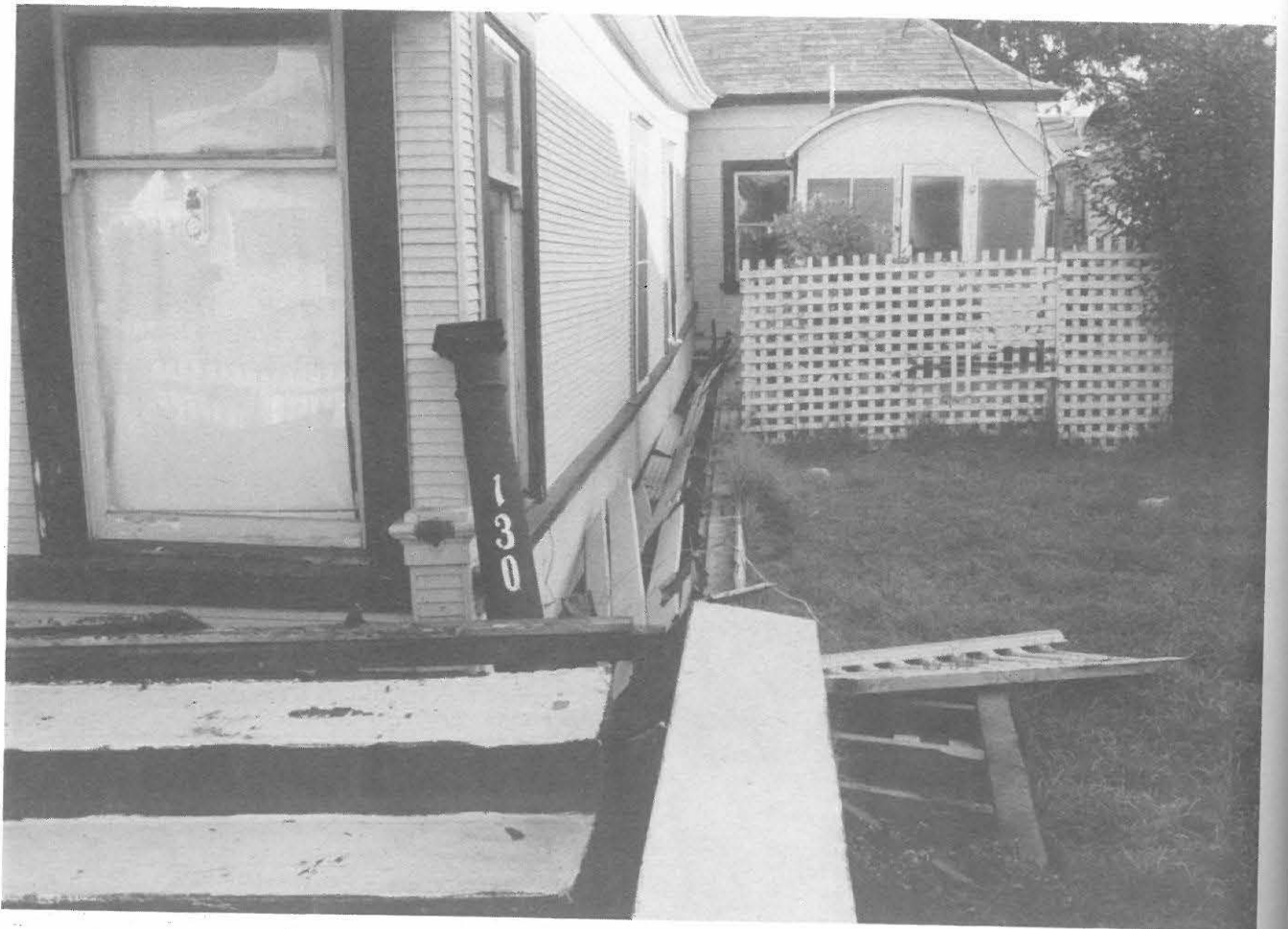
Fig. 3.2 Complete collapse of cripple wall (approx. 2' (64 cm) shift) and destroyed entrance porch due to foundation settlement - 130 Brennan Street in Watsonville
