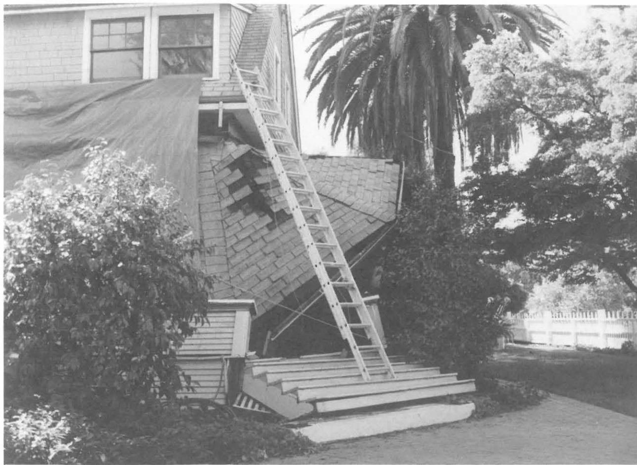
Fig. 3.7 Collapsed porch in an old residence on Main Street in Los Gatos
