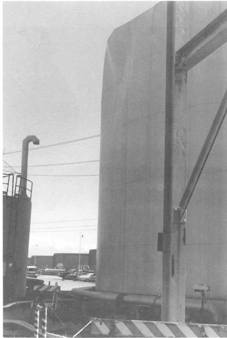
Fig. 5.9 A buckled tank shell - Moss Landing
