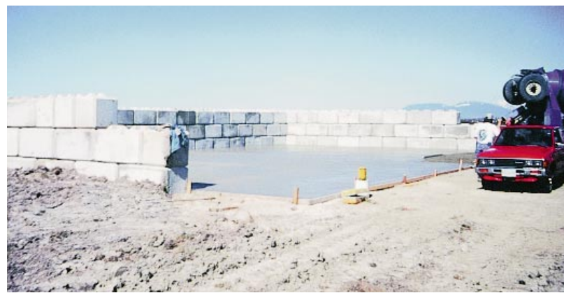
Best practice, like this storage compound under construction, completely isolates the manure.
