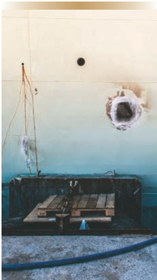
The doubler plate welded to the hull outside the forward AC plant.
