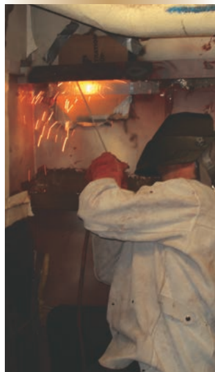
MS Peters doing an overhead weld inside the mechanical workshop to stiffen a structural member of the hull.
