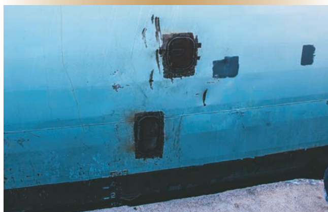
Hull repairs to the outside of the mechanical workshop and the forward engine room. Two doubler plates were welded to the hull of Frederickton by the ship's hull technicians.
