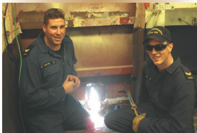
Frederickton hull technicians LS Matthew Boucher and LS Matthew Watson cropped out the damaged section of the hull using oxyacetylene emergency cutting tools.
