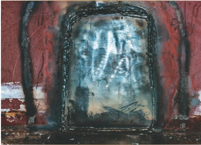
Repair from inside the mechanical workshop, and the deck between the workshop and the forward engine room.
