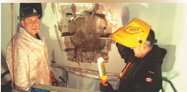
Hull technicians LS Matthew Boucher and AB Lariviere-Lacombe used dogs and wedges to press-fit a doubler plate to the hull prior to welding it in place.
