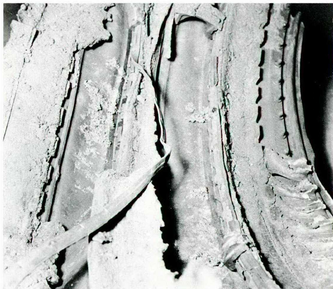
Turbine shroud case showing signs of metal flow from extreme over temp.
