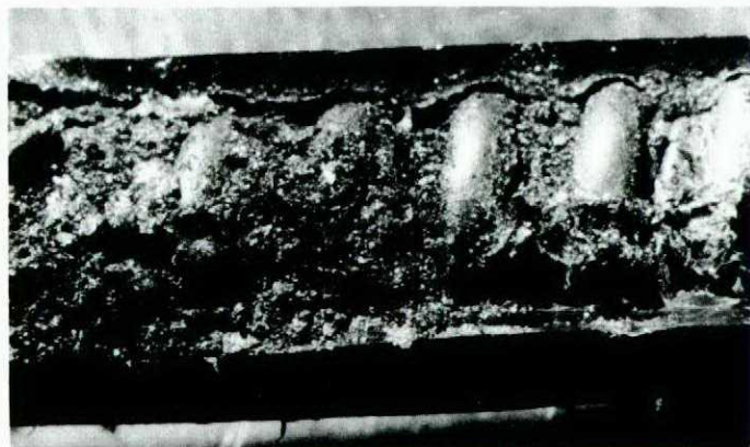
The IGV feedback cable in the teflon liner showing the tightly packed Molykote 77 lubricant.
