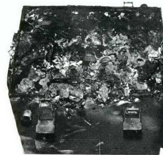
The damage was caused by this battery going into thermal runaway, a result of high ambient temperature and electrical overstressing.
