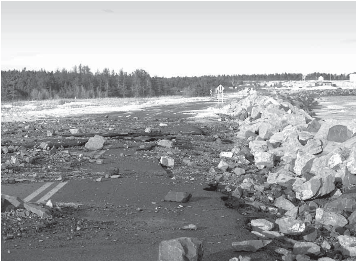
Damages repeatedly sustained on the Route du Banc. Parks Canada / D. Sigouin
