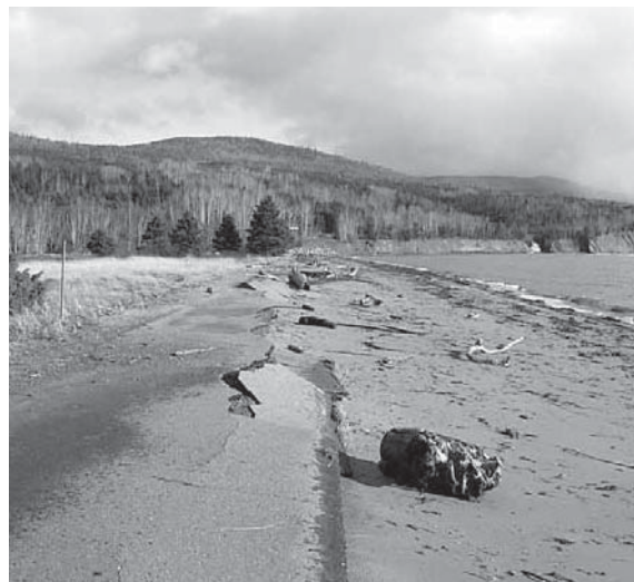
Recurring road damage hindering the visitor experience. Parks Canada
