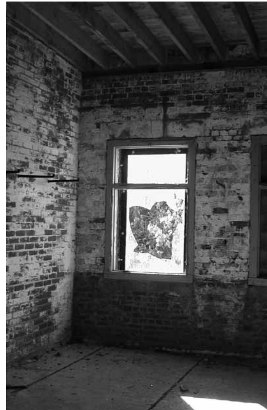
Broken window in the Artificiers Shop. Soonya Quon 2004
