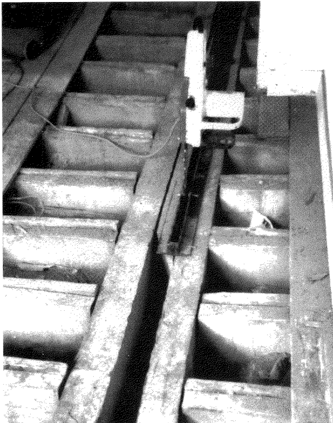
Figure 6. Chainsaw on jig showing partially cut slot in tie beam. Photo: Chris Daniels.
