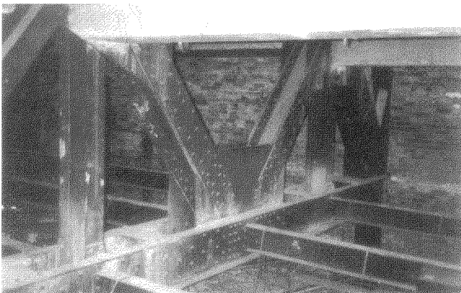
Figure A5. Detail of steel roof truss. The brick casing of the parapet walls, covered in efflorescence, appears in the background. Photo: Khaled Ibrahim.
