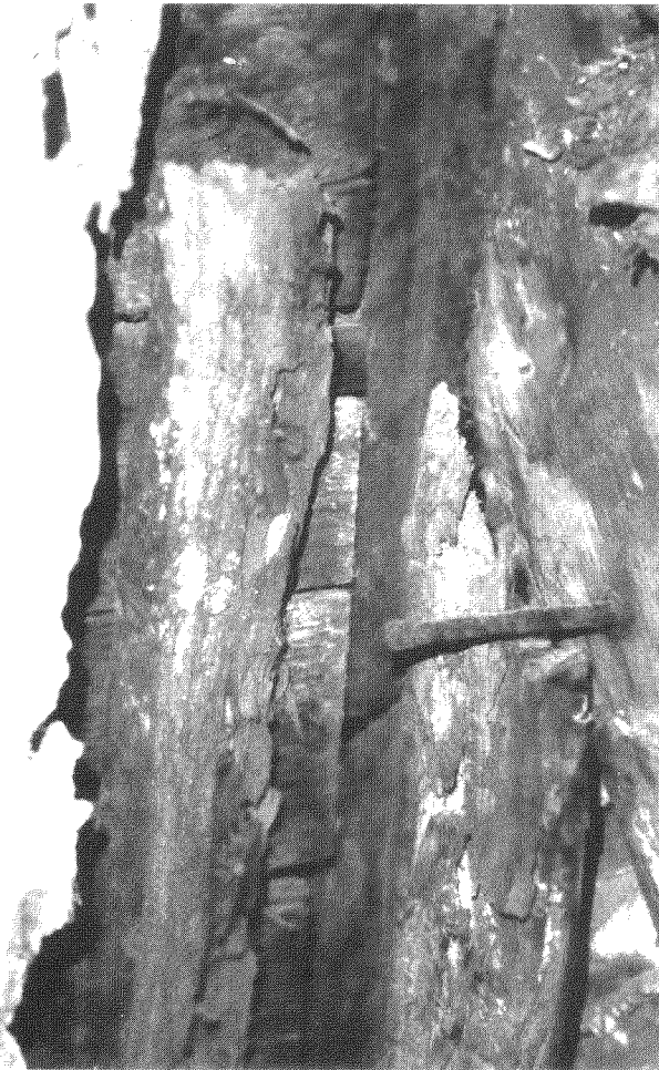
Figure 10. Extent of missing wood from rafter. Remnant of rafter resting against roof boarding. Note nail at right is 150 mm long and was used to attach joist to rafter. Photo: Chris Daniels.
