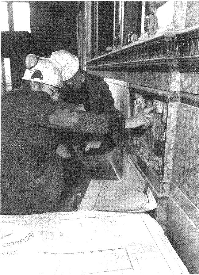
Figure 6. Once the test indicated that the procedure located the plaster adhesive patches with 90% accuracy, the survey continued.
