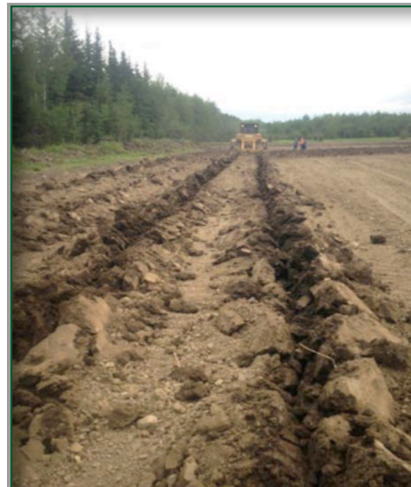
Figure 5a. Bulldozer with two straight ripper attachments on extremely compacted and dry soil
