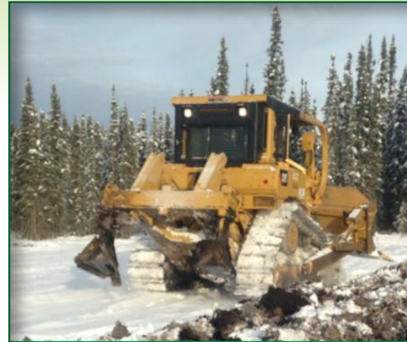
Figure 1a. A winged subsoiler in the outside pockets of a multi-shank toolbar attached to a bulldozer
