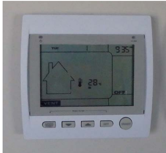
Figure 20: Image of an installed advanced controller in a LEEP field trial home. Photo credit: Gio Robson
