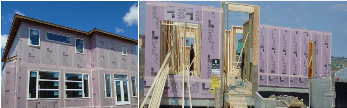
Figures 9 & 10: Pictures of two Manitoba LEEP field trial homes under construction. Photo credits: Figure 9: Gary Proskiw, Figure 10: Gio Robson
