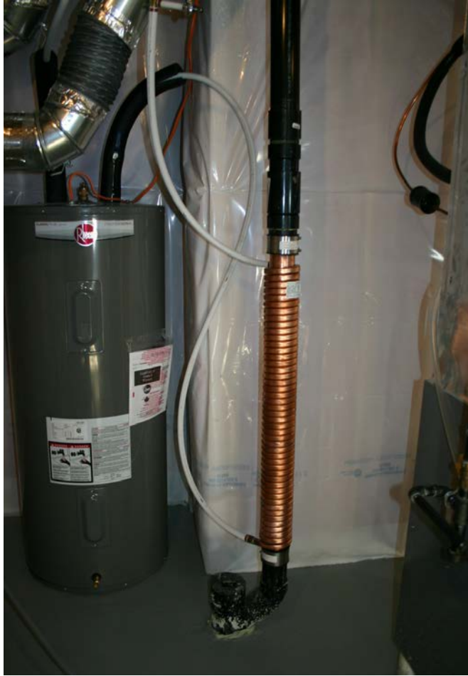
Figure 21: Installed Drain Water Heat Recovery system in LEEP field trial home. Photo credit: Gio Robson
