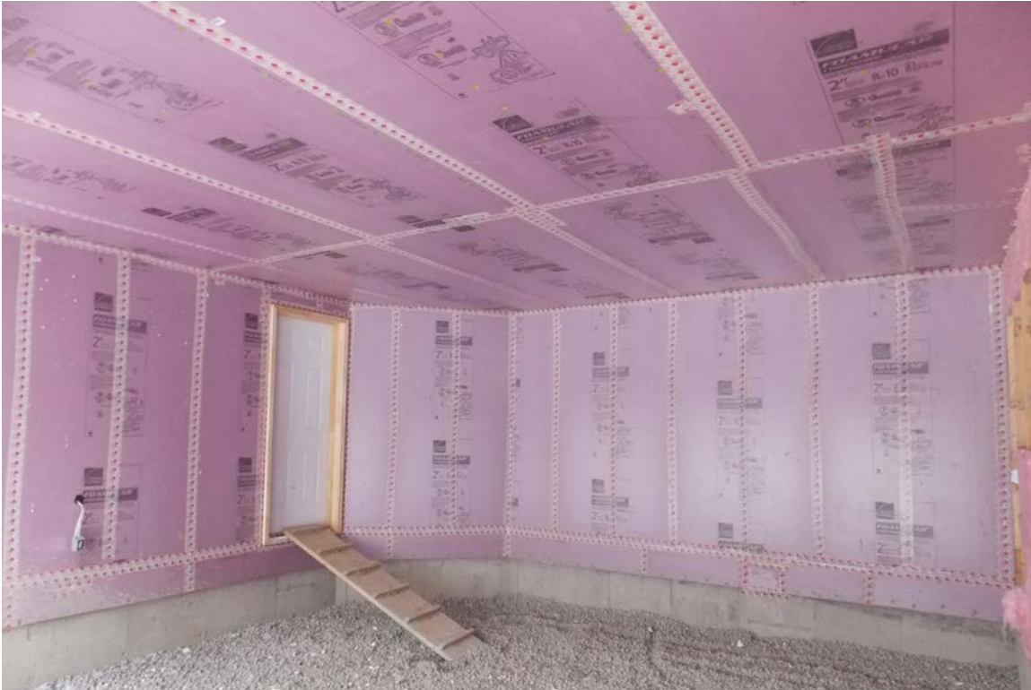
Figure 14: Example of foam board sheathing applied to the underside of a floor above a garage. Photo credit: Owens Corning Canada
