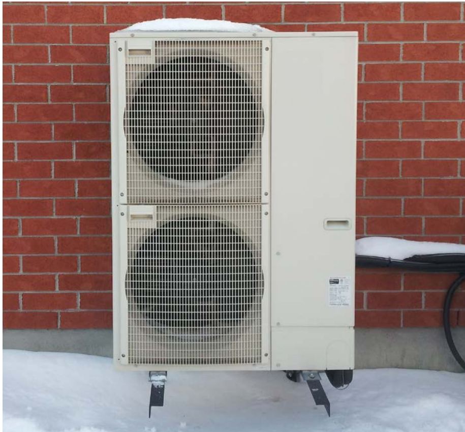
Figure 23: Image of an installed CCASHP at the Canadian Centre for Housing Technology, Ottawa. Photo: Natural Resources Canada
