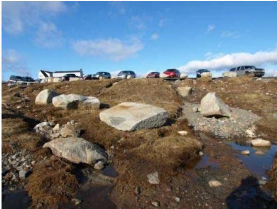
Figure 3-4: (Top) Erosion around east side of restaurant parking lot. (Bottom) All the large rocks shown were moved, some on top of paths.
