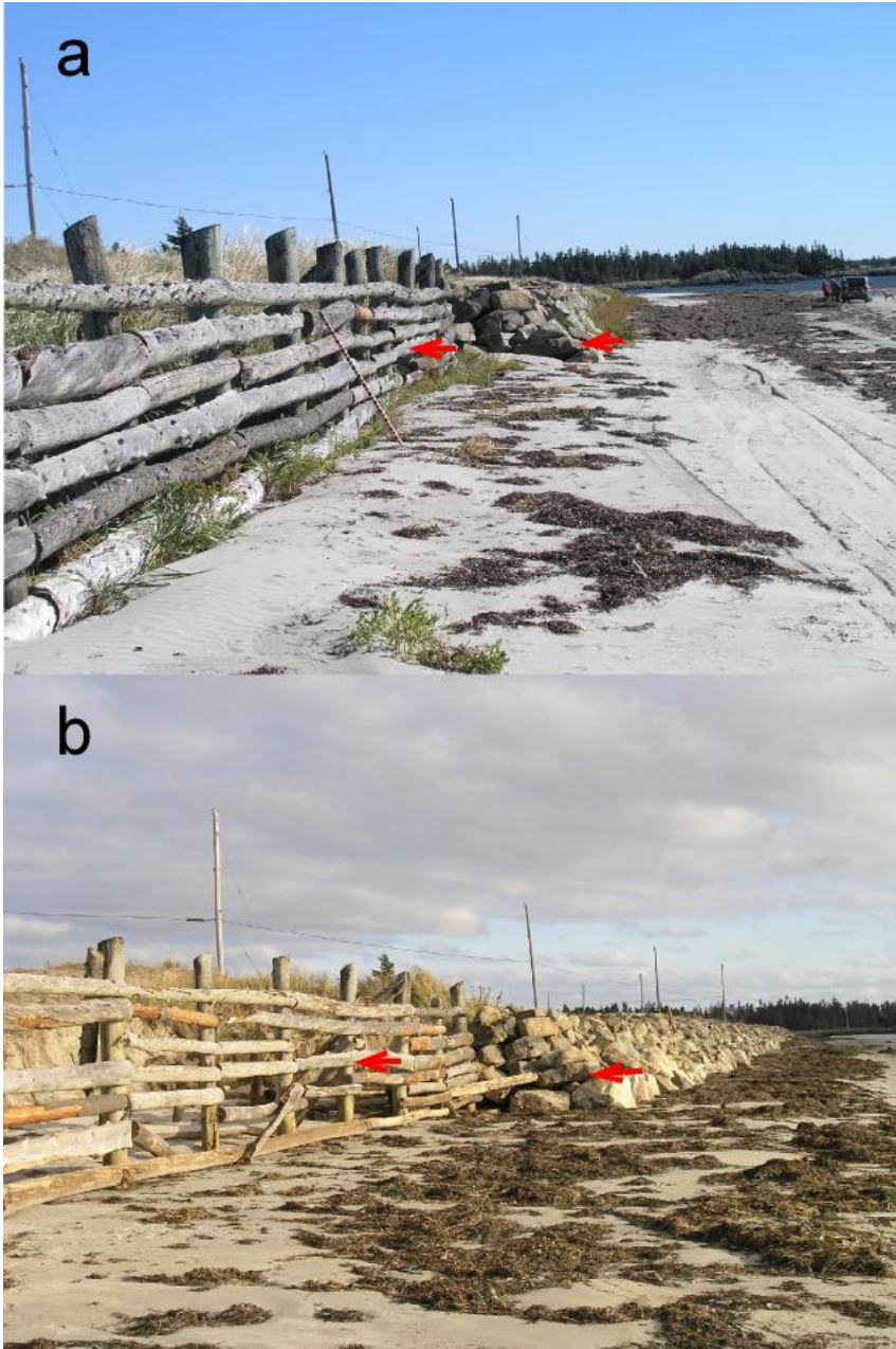
Figure 36. View of the fence and rock wall at the east end of Crescent Beach at Line 38 on (a) Oct. 7, 2007 and (b) Nov 9, 2007 showing a similar depth of wave scouring by waves during Noel at the two interfaces. Arrows mark the same location on each photo. The survey pole against the fence in (a) is 1.54 m long. (photo PA70205 and PB090685, R. Taylor)
