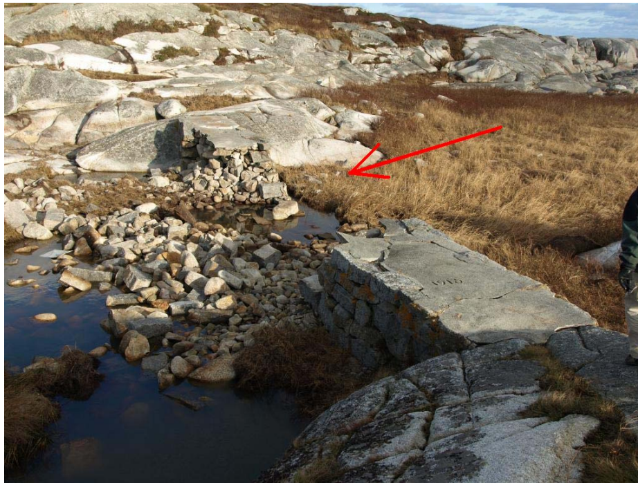
Figure 3-5: (Top) Breakwater (arrow) after Juan, with no significant damage. (Bottom) After Noel, with about half of it totally destroyed. The breakwater was built over 100 metres from the ocean and has remained undamaged for 92 years.
