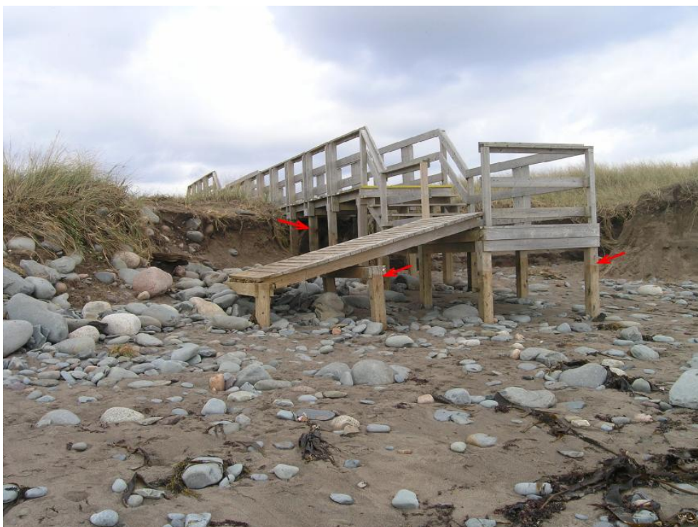
Figure 16. View of boardwalk just west of Line 303 where waves scoured a significant portion of beach and dune as indicated by the former ground surface marked by a stain line (arrows) on the support posts (photo PB050359, R. Taylor).
