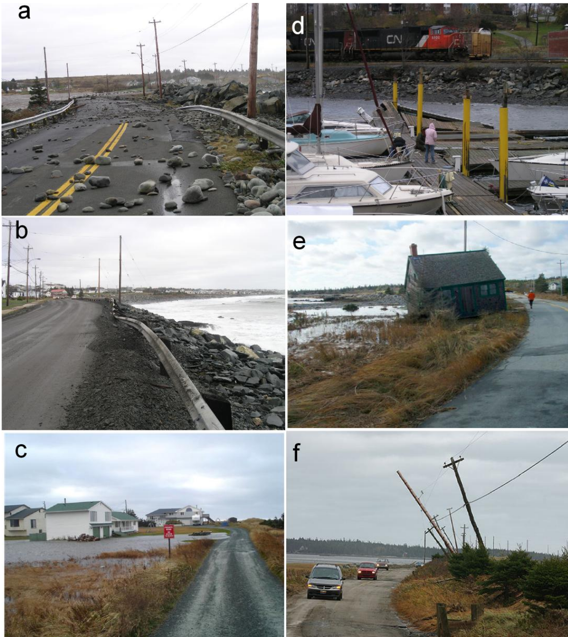
Figure 4a. Examples of wave impacts from Noel to coastal infrastructure along the Atlantic coast of Nova Scotia (a) rock debris and damage to pavement Cow Bay Road; (b) bent guard rail and debris, Eastern Passage Shore Road; (c) flooding at Wyndenfog Lane, Lawrencetown Beach (Betty, Houghton); (d) damage to wharves and sailboats Halifax Harbour; (e) floating structures, West Berlin, N.S. (Kirsty Toussignant); and (f) downed power lines Crescent Beach Lunenburg Co. (Bridgewater News). All photos were taken on November 4, 2007 by R. Taylor (GSCA) unless noted.
