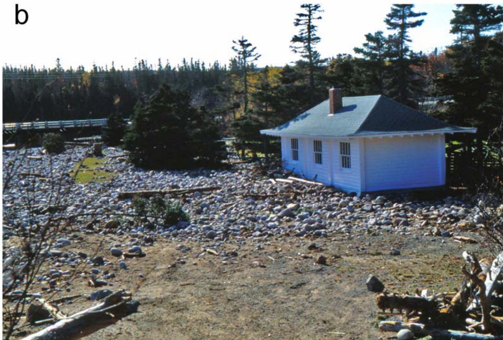
Figure 38. Views of the damage caused by the storm surge October 26, 1983. (a) cobbles and debris carried up the smooth grass slope to 4 and 7 m elevation on BBCB and (b) cobbles and flotsam were carried landward against the picnic shelter and base of the highway along BBCB-south.
