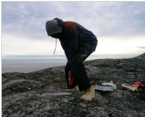
Adule Chris drills into solid bedrock to prepare for the GPS medallion installation.
