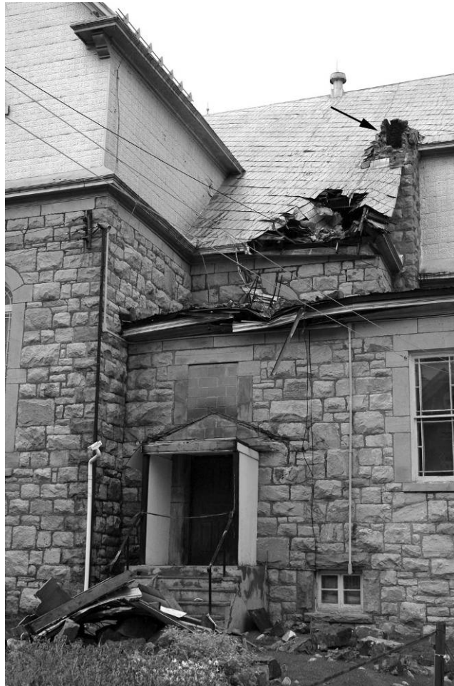
Figure 2-18 Damage to l'Église de la Visitation, Gracefield, Quebec, from the June 23, 2010, earthquake. Arrow marks the location of the chimney which toppled and damaged the roof and an entranceway cover while falling to the ground (Photograph: Greg Brooks).
