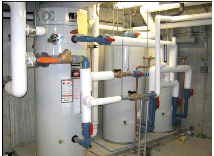
Figure 6 Gas-fired water heater and storage tanks (Credit: L'OEUF s.e.n.c.)
