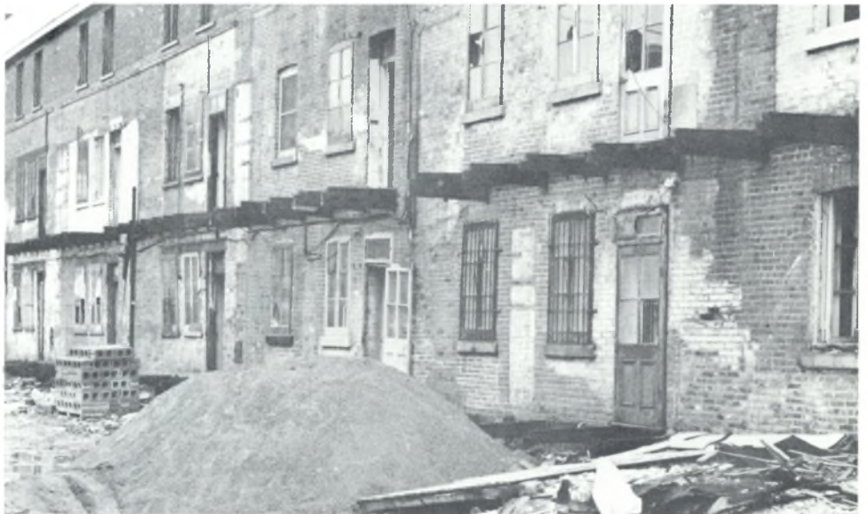
One of the first steps in this rehabilitation program in Montreal was the removal of back sheds, lean-to's, outbuildings and old fencing to eliminate obvious fire and health hazards.
