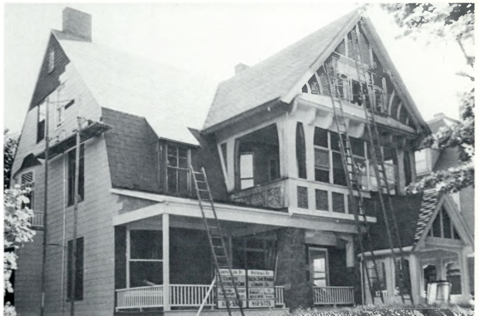
Rehabilitation of a typical Boston "three-decker" — a wood-frame building containing three apartments. The building is being rehabilitated inside and out as part of the Boston Redevelopment Authority's Washington Park Urban Renewal Program.
