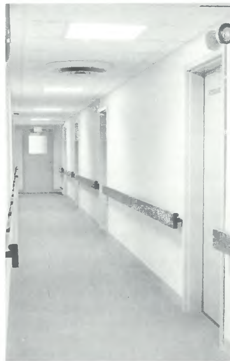
Corridors are equipped with handrails and low pile carpeting which are of benefit to both the handicapped and the elderly.
