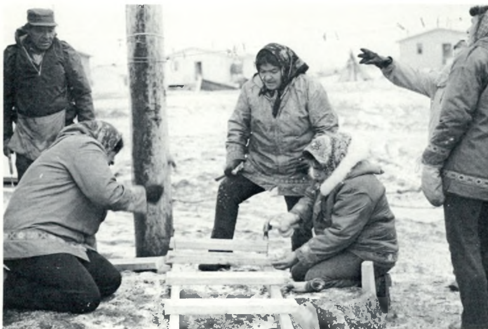
Both men and women take part in the repair program. Native people in Fort George, Que., building a ladder to make roof repairs.
