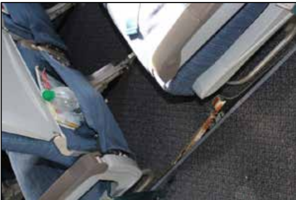
Figure 10. Floor damage forward of passenger seat 31D
