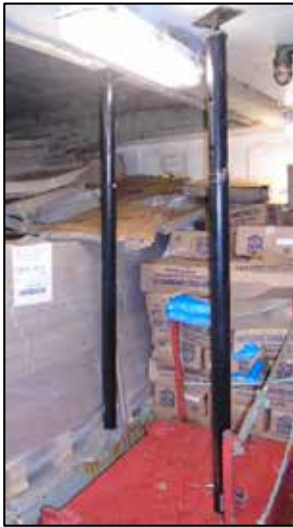
Figure 3. Jack posts used to secure hatches (Source: Nataaaqnaq Fisheries)
