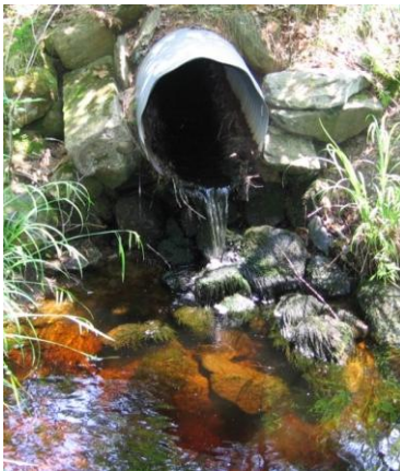
Impassable culvert due to the outlet drop at the Canning Field Road crossing of Rogers Brook, Kejimkujik. Oliver Woods.
