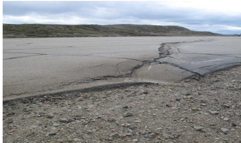
Asphalt depression caused by localized permafrost melting, Iqaluit airport
