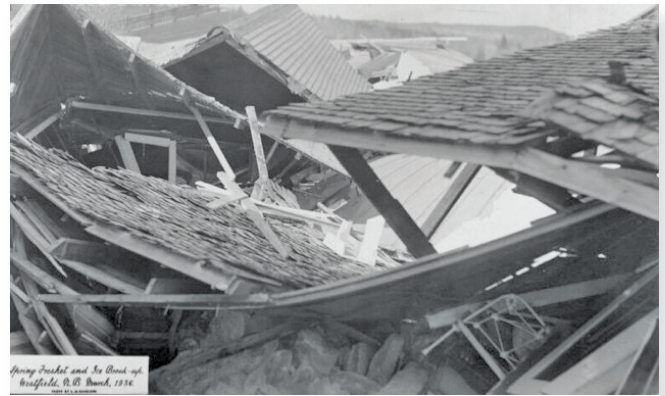
Figure 2: Infrastructure damaged in Westfield by a river ice jam on the Lower Saint John River in the Spring of 1936 Town of Grand Bay-Westfield
