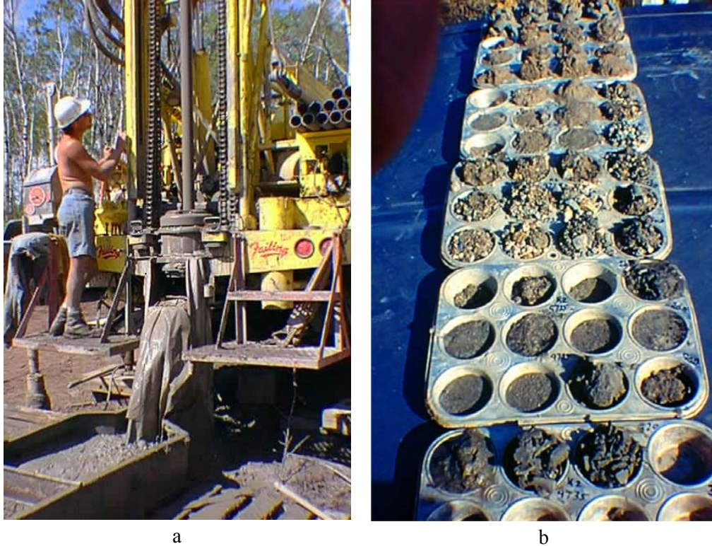
Figure 17: a) Mud rotary drilling rigs are a cost effective method for subsurface sampling of fine-grained, matrix-rich tills; b) Cleaned samples collected from a mud rotary drilling rig range from clays and silts (cuttings), fine sands, sands and gravels, to fine-grained till (cuttings; extreme back).
