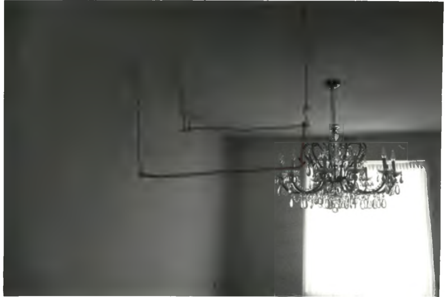
NOTE THERMOGRAM LOCATION AND PROBLEM AREA
