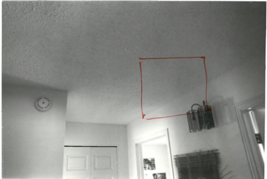
NOTE THERMOGRAM LOCATION AND PROBLEM AREA
