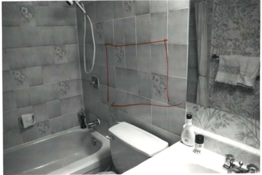
NOTE THERMOGRAM LOCATION AND PROBLEM AREA
