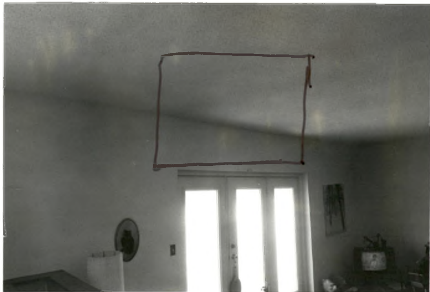
NOTE THERMOGRAM LOCATION AND PROBLEM AREA
