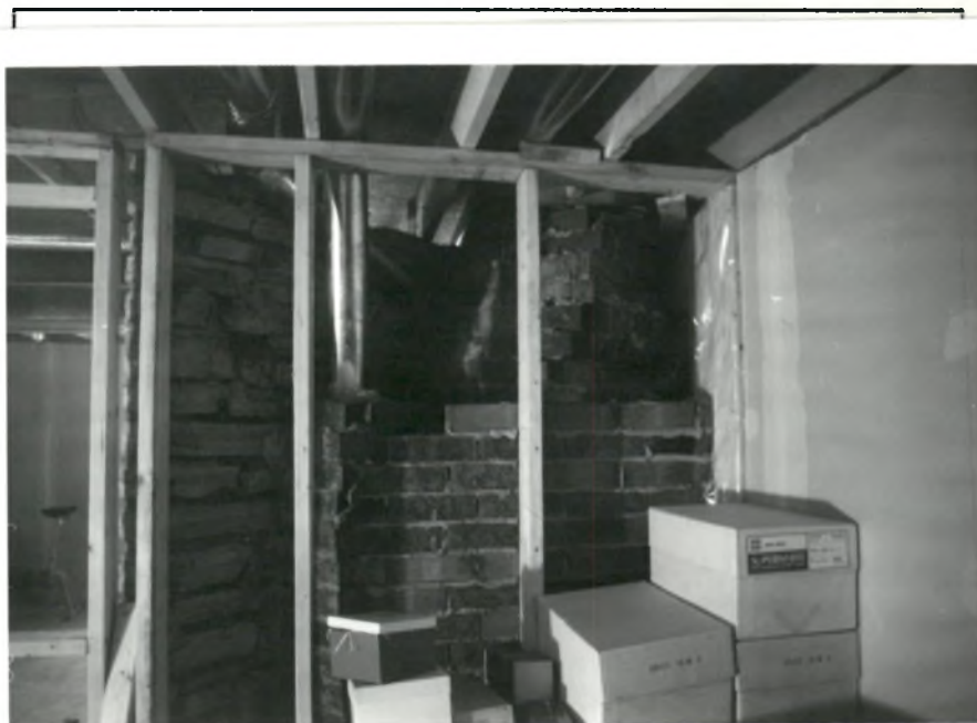
NOTE THERMOGRAM LOCATION AND PROBLEM AREA
