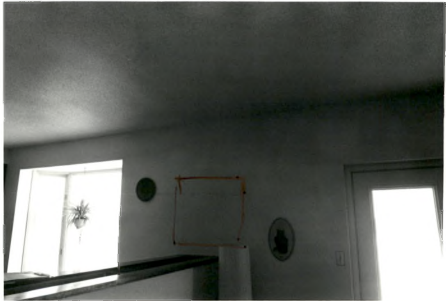
NOTE THERMOGRAM LOCATION AND PROBLEM AREA
