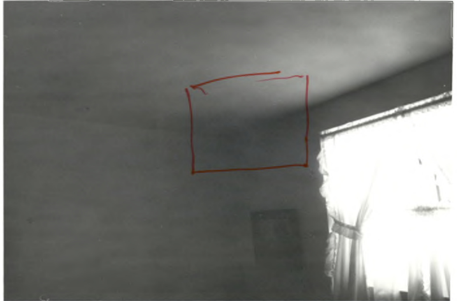
NOTE THERMOGRAM LOCATION AND PROBLEM AREA
