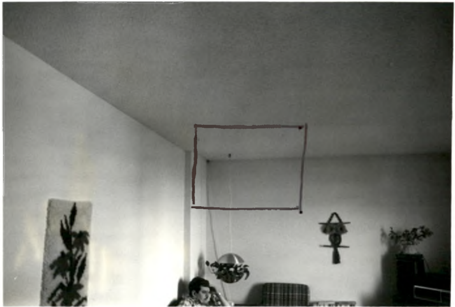
NOTE THERMOGRAM LOCATION AND PROBLEM AREA
