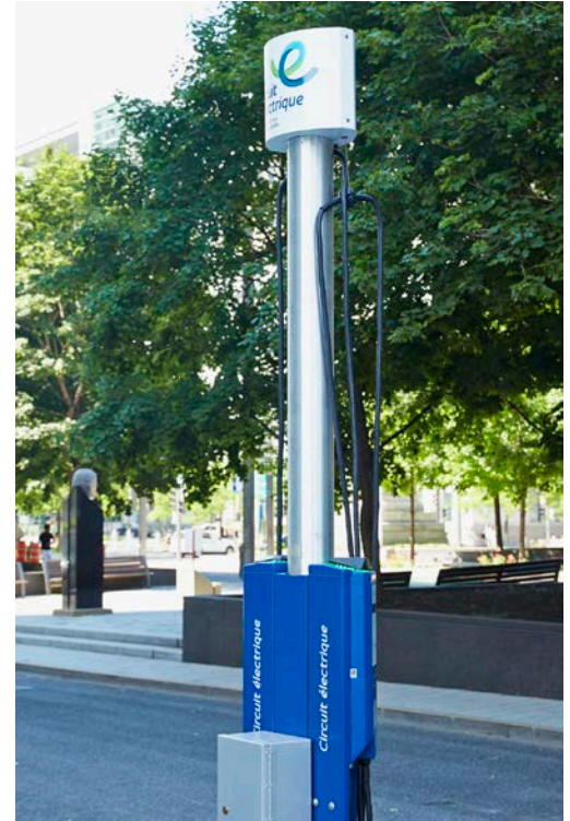
Over 180 municipalities, institutions and businesses partner with Hydro-Québec to install EV charging stations.
