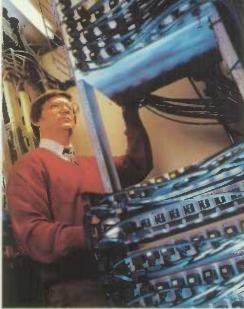
A technician of Bell Canada attends to the installation and maintenance of the telecommunications equipment at Sunnybrook Medical Centre in Toronto, Ont.
