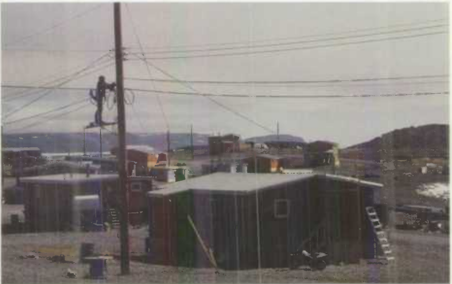
Communications equipment in Holman Island, NWT.
