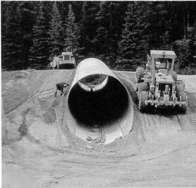
Installation of an underpass to facilitate animal movement, reduce road kills, and improve public safety, Banff National Park
