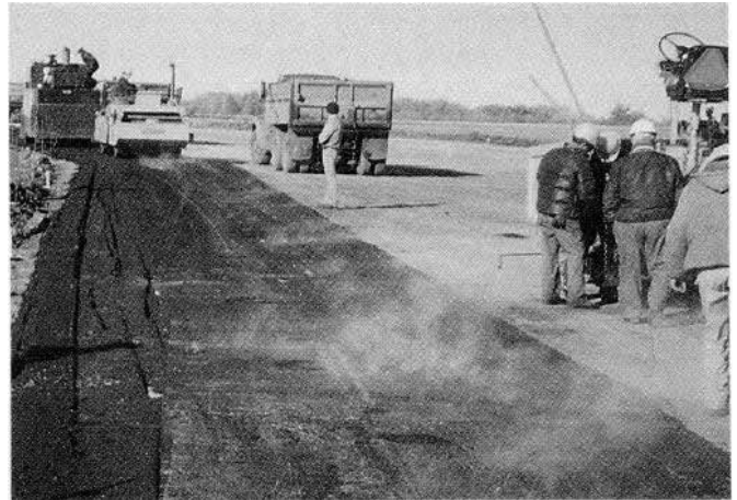
Airport runway construction, following an initial assessment of the project by Transport Canada
